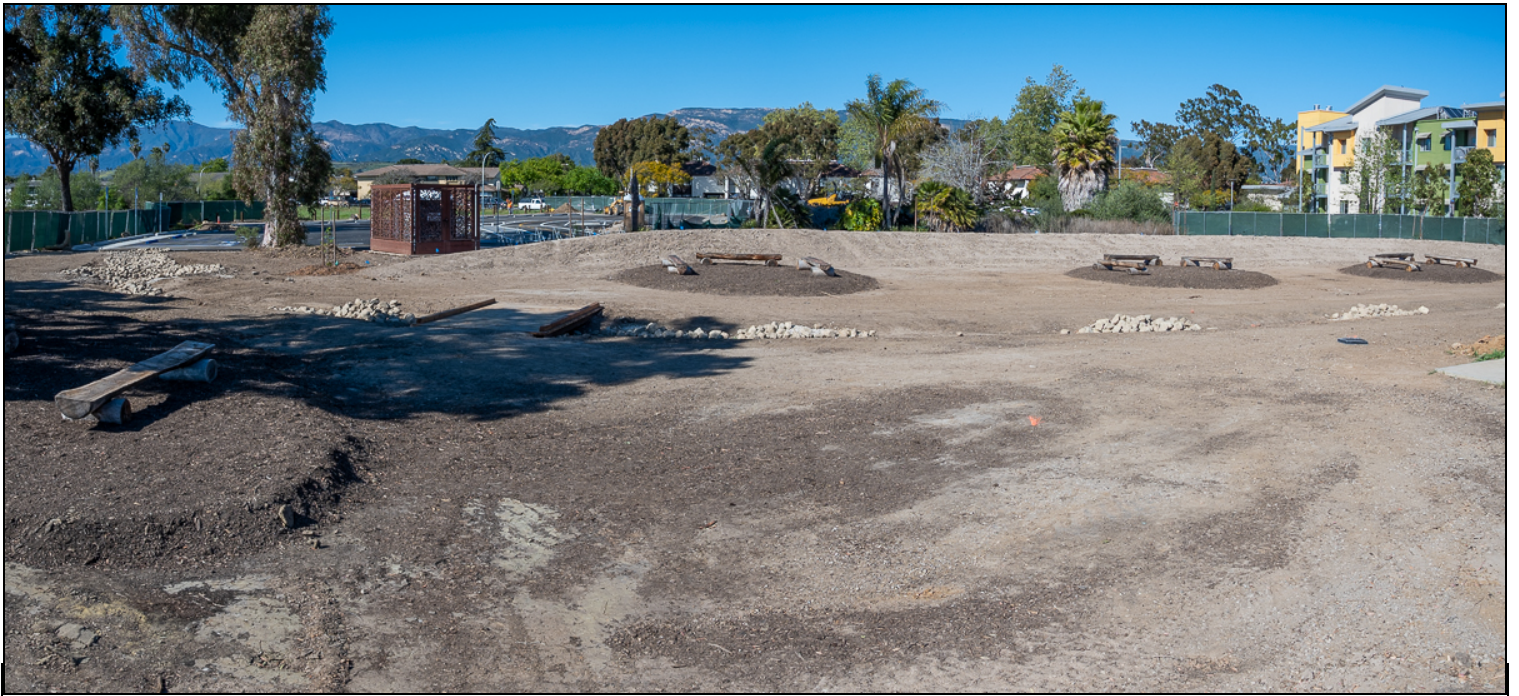
This open space will be planted with rhizomatous native saltgrass ( Distichlis spicata ), which will spread and form a lawn.
