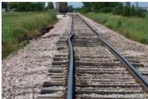
(a) Sunkink misalignment
