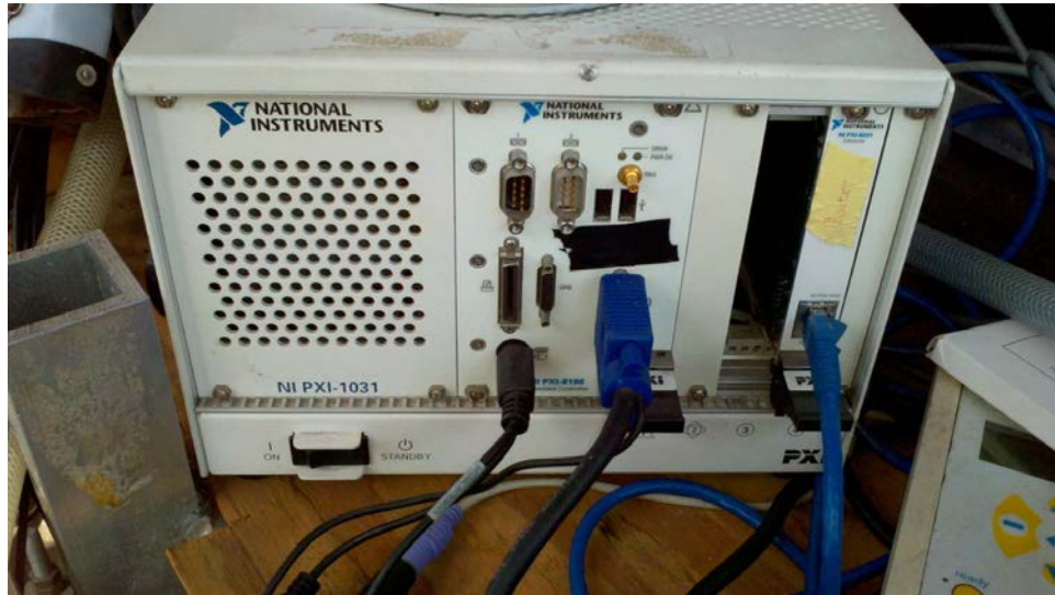
Figure 6-12: Data Storage PXI Chassis
