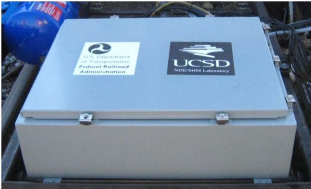
Figure 6-6: Weatherproof NEMA Box for Outboard Analog Electronics
