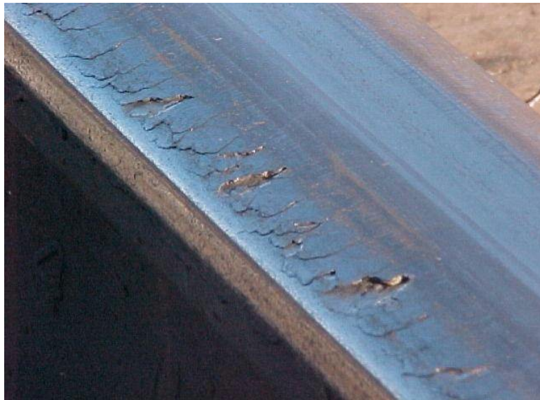
Figure 3-11: Rail Surface Checking and Flaking
