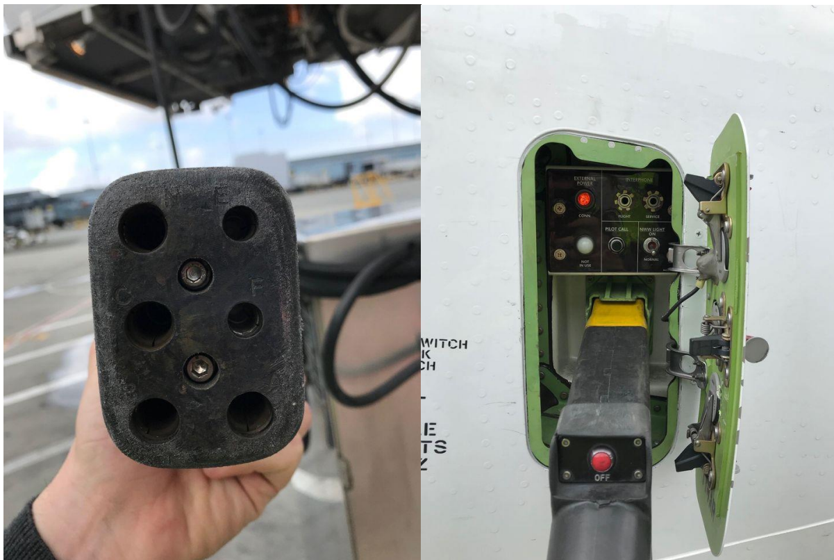
Figure 35: GP connector and receptacle at SFO international airport (Achatz Antonelli, 2019)
