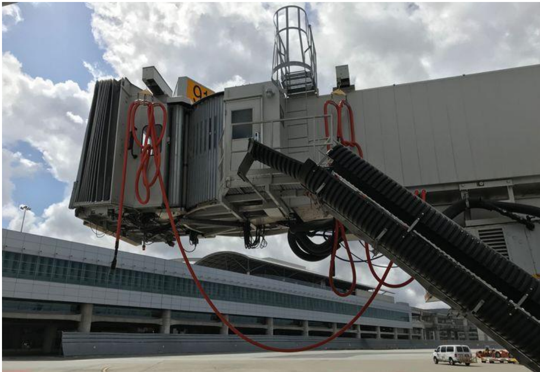
Figure 34: Jet bridge with GP cable connected to a pulley system at SFO international airport (Achatz Antonelli, 2019)
