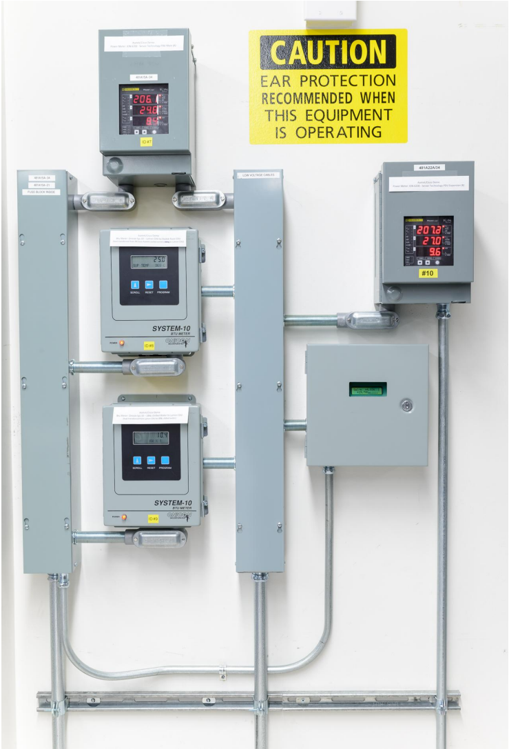
Figure C-1: Installed Electrical And Btu Metering
