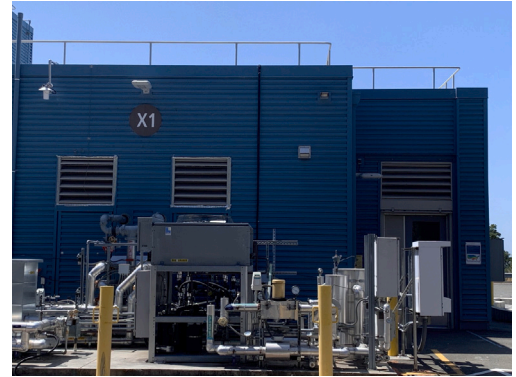
Fig. 3. Outside view of the chiller and chilled water system of the FLEXLAB test cell.
