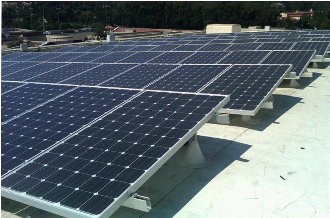
Figure 22 Solar panels on Ackerman Union's roof
