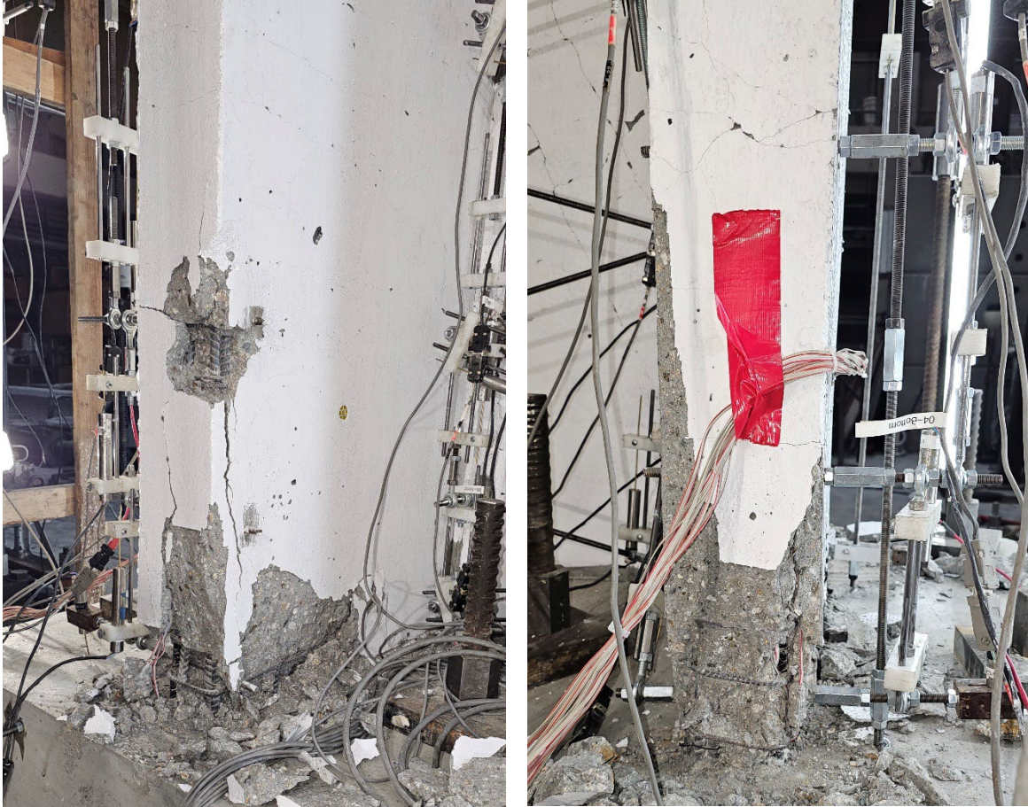
Figure 5-5: East flange edge (left), West flange edge (right) after inelastic ramp-down cycles of WLP, CW-2
