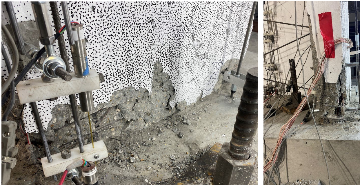
Figure 5-8: West flange after the completion of WLP, CW-2
