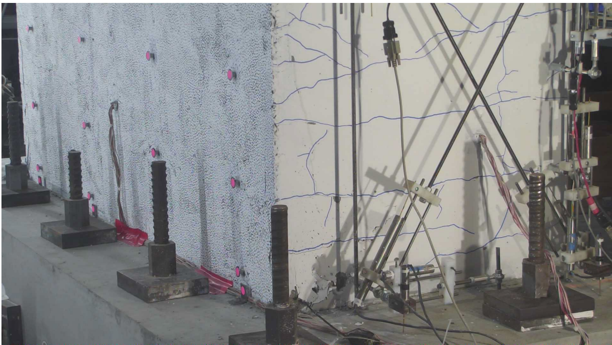
Figure 4-2: Damage state of the East flange and the web after two cycles at 1.5% hinge rotation demands (at zero loads)
