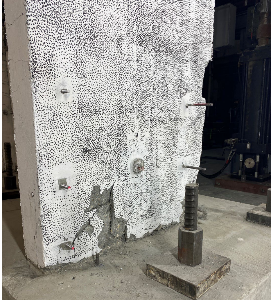
Figure 6-9: Damage state of the west flange after the completion of testing, CW-3
