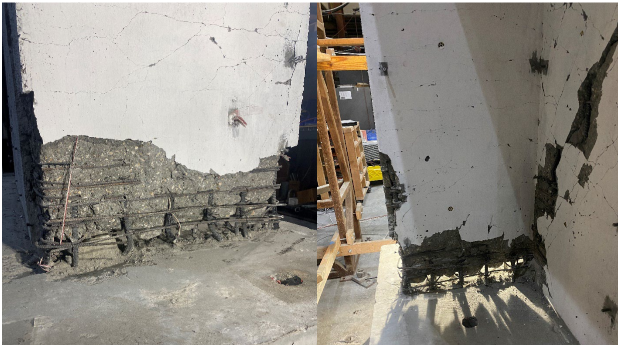
Figure 6-1: Damage state of the east flange after the completion of testing, CW-2
