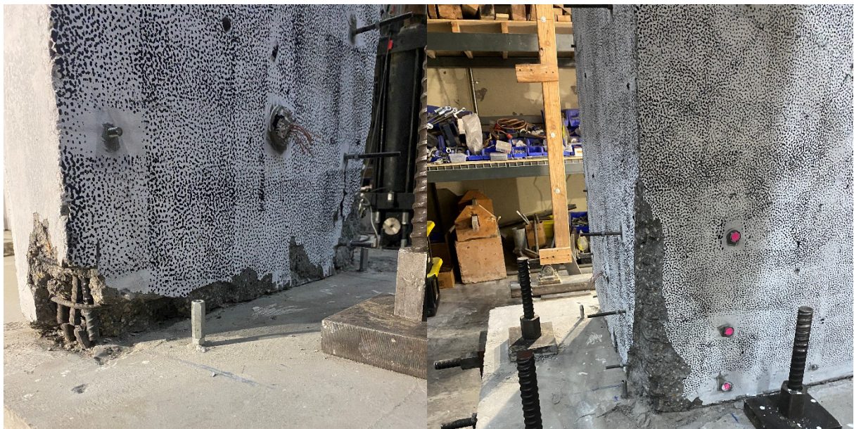
Figure 6-11: West flange edge (left) and west flange corner (right) after the completion of testing, CW-4
