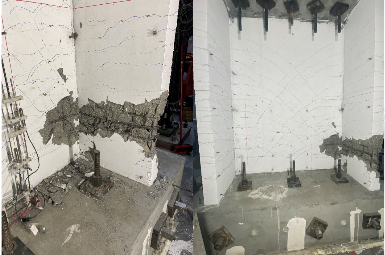
Figure 4-7: Inside surface of West flange (left) and the web (right), after the test
