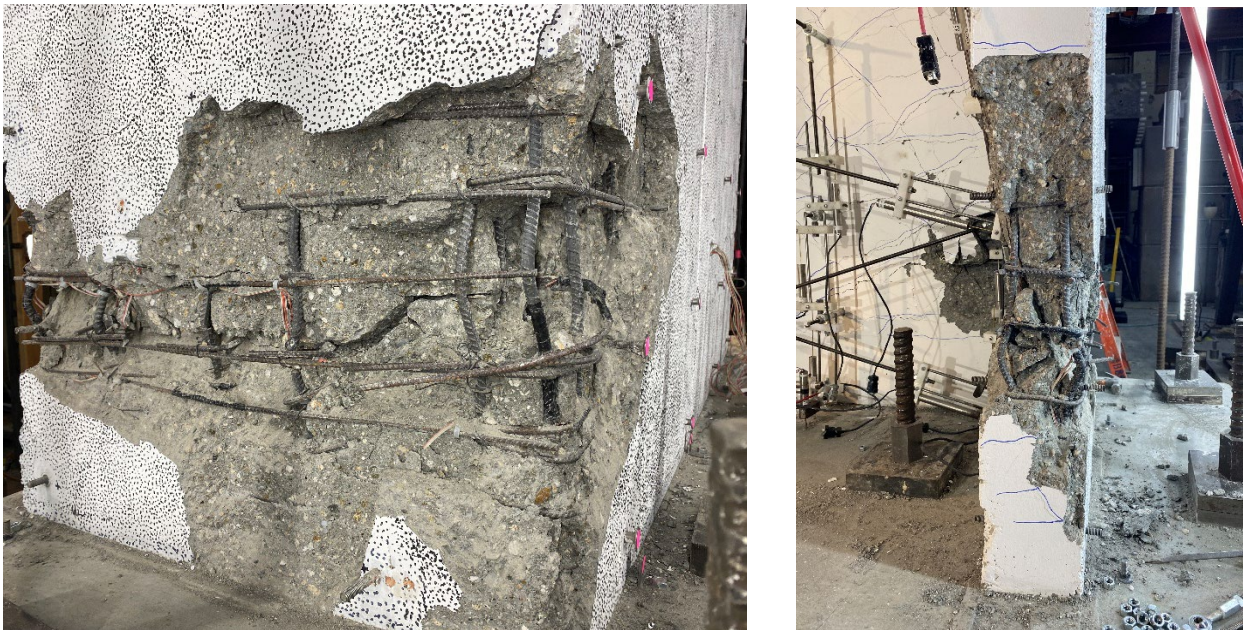
Figure 4-6: West flange close-up pictures after the test
