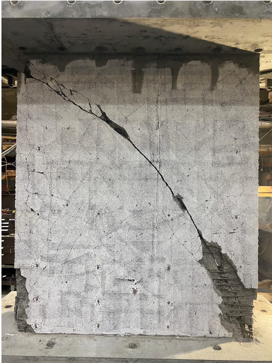
Figure 6-2: Outside surface of the web after the completion of testing, CW-2
