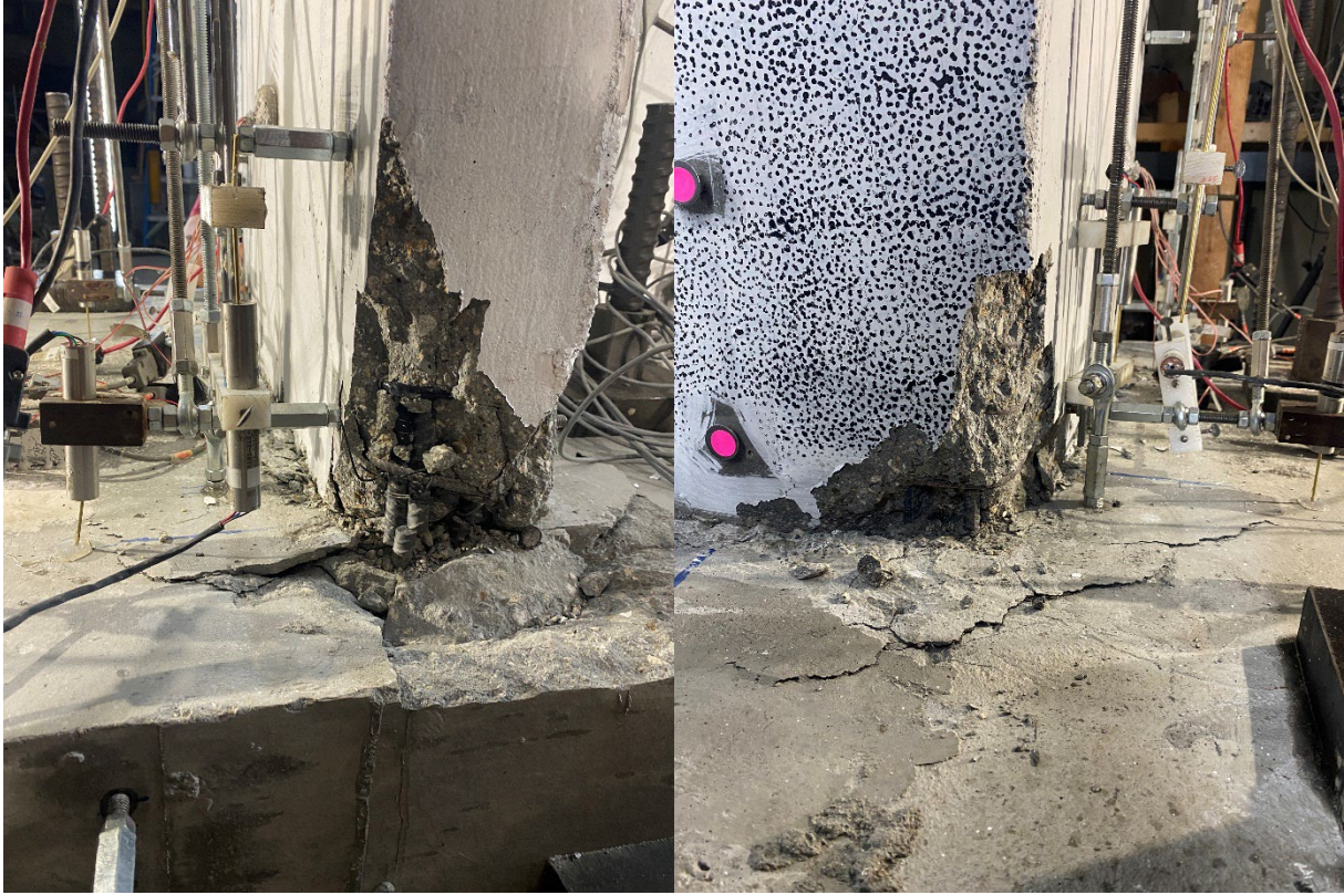
Figure 6-10: East flange edge (left) and east flange corner (right) after the two cycles applied at \pm 0.9\% IP hinge rotation demands, CW-4
