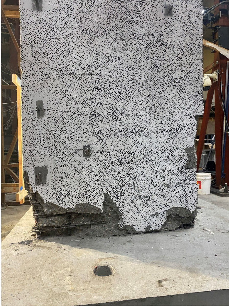
Figure 6-4: Damage state of the west flange after the completion of testing, CW-2
