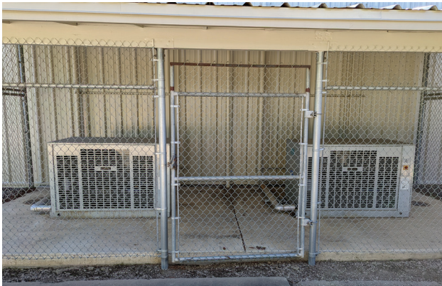
Figure 5.42. Secured condenser units for walk-in freezer are protected from the elements.
