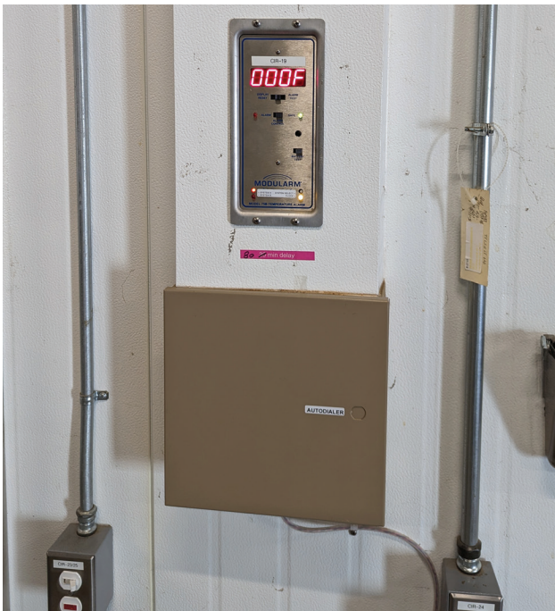
Figure 5.41. Freezer temperature control panel.
