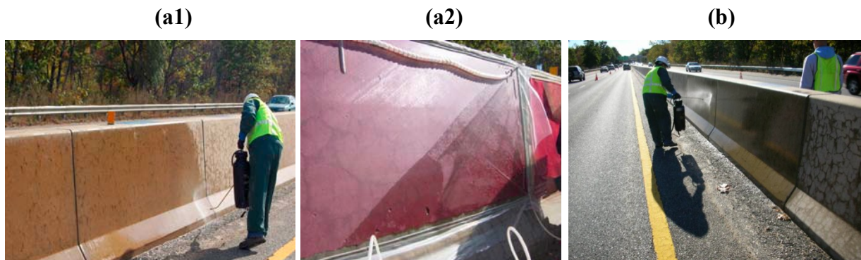
Figure 4-4. (a1) Topical and (a2) vacuum application of lithium nitrate solution on ASR-affected highway barriers [124]. Folliard et al. [124] found the topical and vacuum applications of lithium nitrate was ineffective in reducing the reactions due to lack of penetration of the solution. (b) Topical application of 40 percent-Silane Solution (solvent-based) to ASR-affected highway barrier in Massachusetts [125]. Penetration depths of silane solutions are typically measured to be less than 5 or 6 mm. Generally, this depth is adequate for preventing water from entering the concrete while
