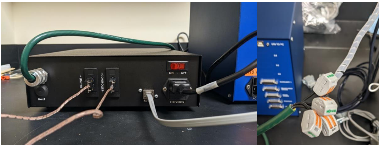
Figure A.6: Left: Back-view of the temperature controller box with all the electrical connections attached. Right: Lever-lock connectors.
