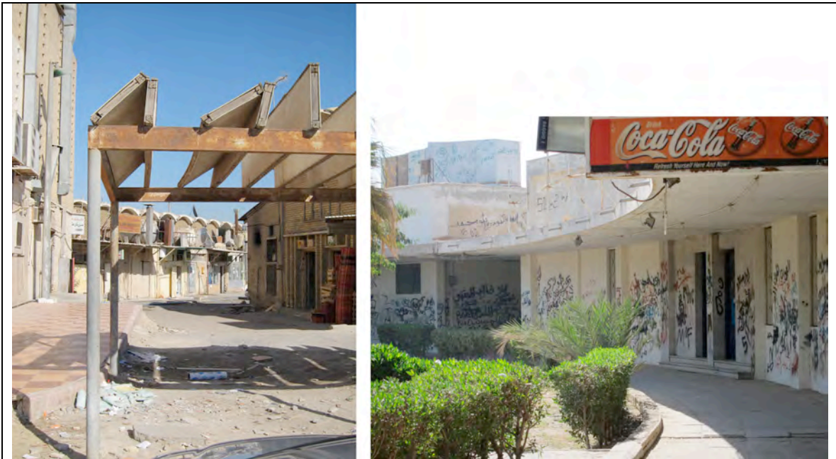
Figure 15. The Vandalized and derelict current state of the Ahmadi shopping center. (Source: Author)
