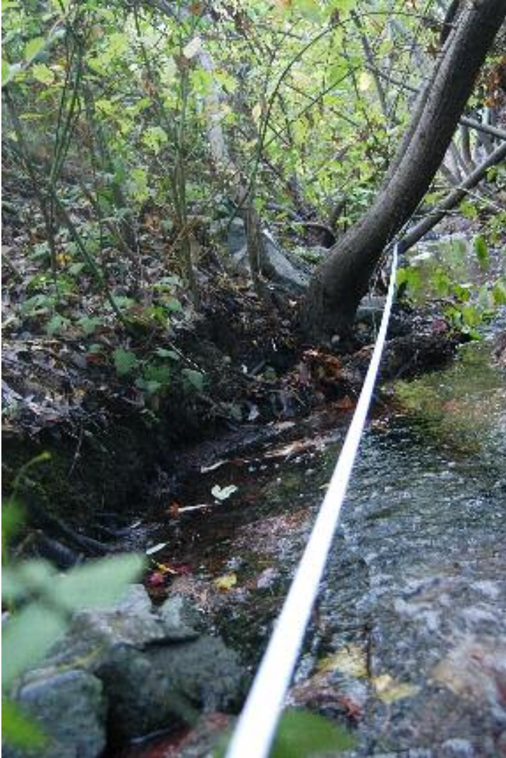
Figure 9: Erosion of Left bank (Station 1+03 facing downstream); Dec 2005
