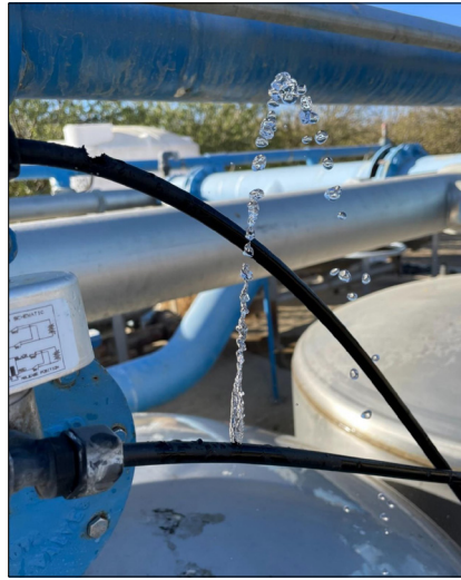
Plate E. Roof rat chewing damage to irrigation tubing. Source: Juan Ayala Cruz, California Department of Food and Agriculture.
