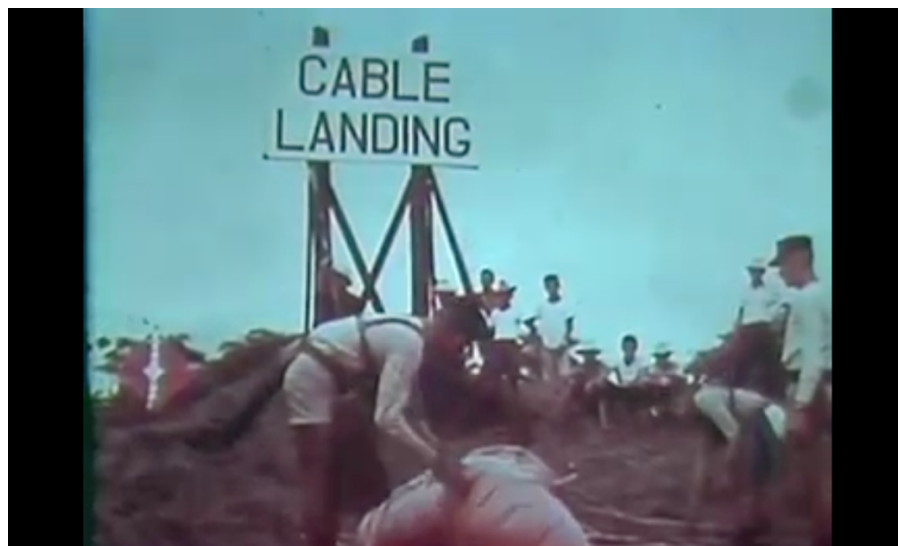
Figure 16: Cable Landing point at Baler, PH, from AT&T Documentary on C.S. Long Lines . 122
