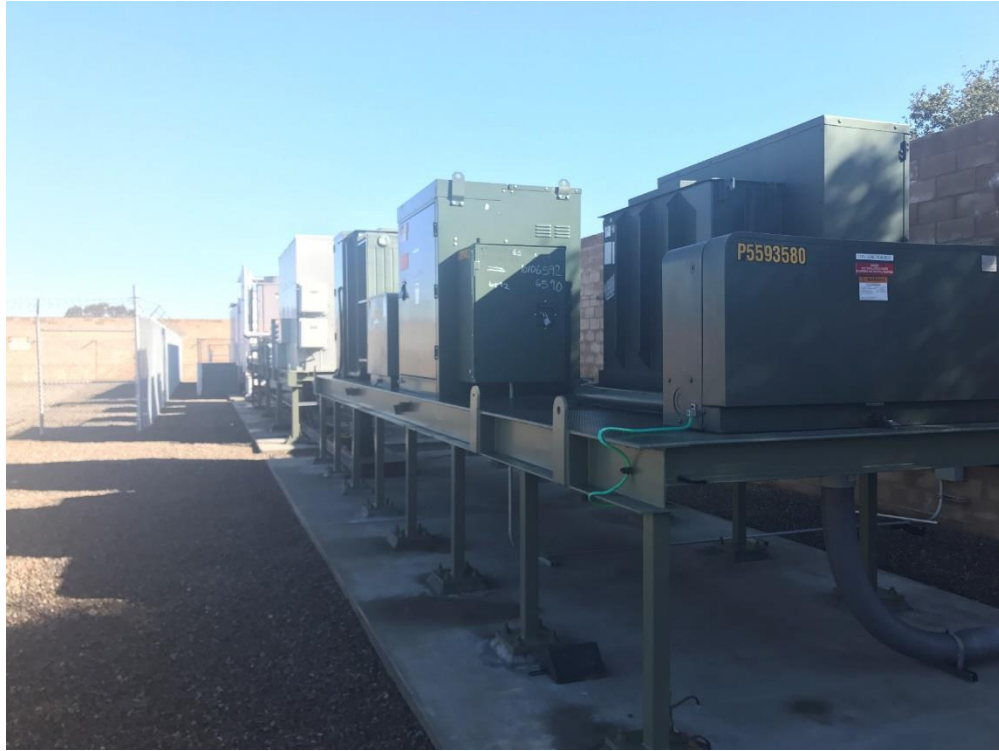
Figure 45. UCIMG battery energy storage system.
