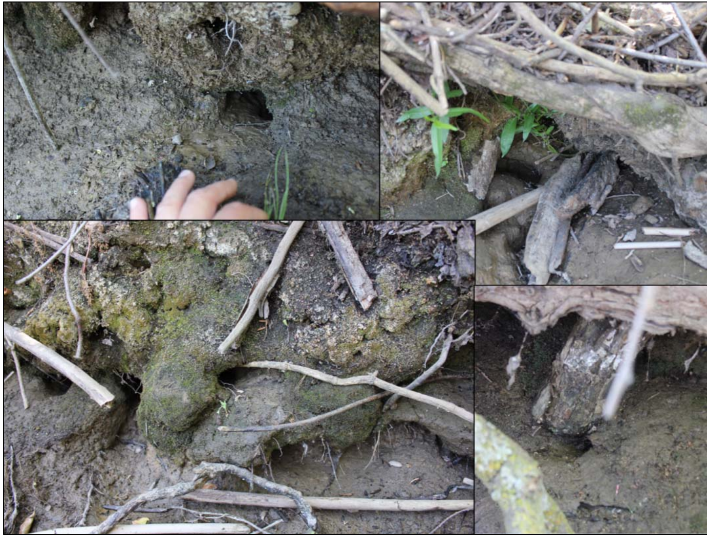
Figure 3-150. Photos taken on 6/1/12, the day after completion of the flow test. The waterside burrows are photographed and observed to have stopped flowing.
