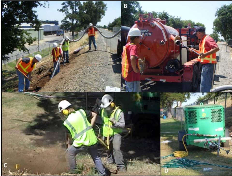
Figure 2-24. Construction equipment used during excavation. A) hand excavation with vacuum to remove spoils; B) a vacuum trailer; C) air knife used to excavate around live roots; D) 375 CFM compressor to run the air knife.
