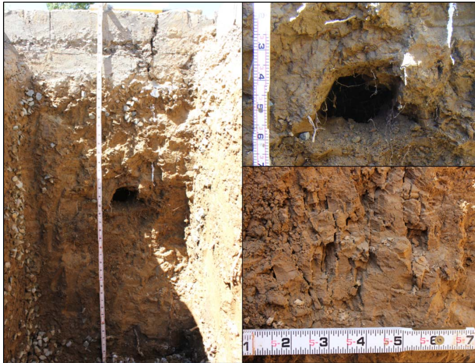
Figure 3-177. View north of tree trench end wall at Station TT 0 showing a burrow (2 feet deep) and a series of vertical tension cracks along bedding planes of Material 2 (thinly bedded silt).
