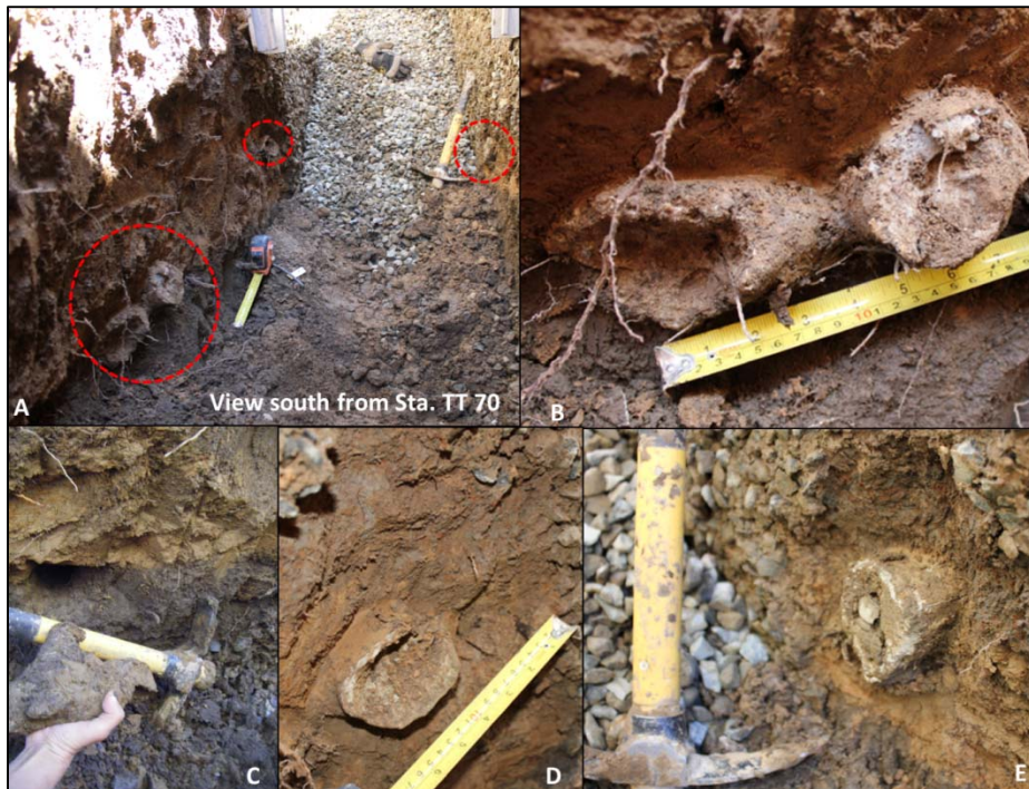
Figure 3-180. Patched burrows Station TT 70 to 73. A) overview of patched burrows, B) and C) Initially intact burrow patch is removed and viewed; D) intact landside burrow patch; E) intact waterside burrow patch.
