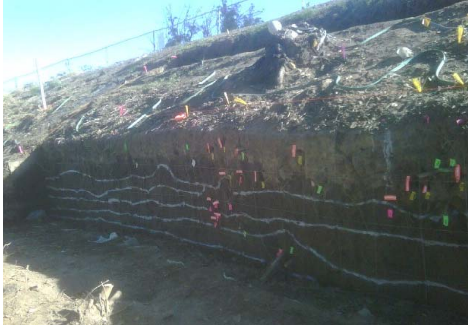
Figure 2-78. View looking southeast at the trenches following excavation of the downhill wall of the lower stump trench.
