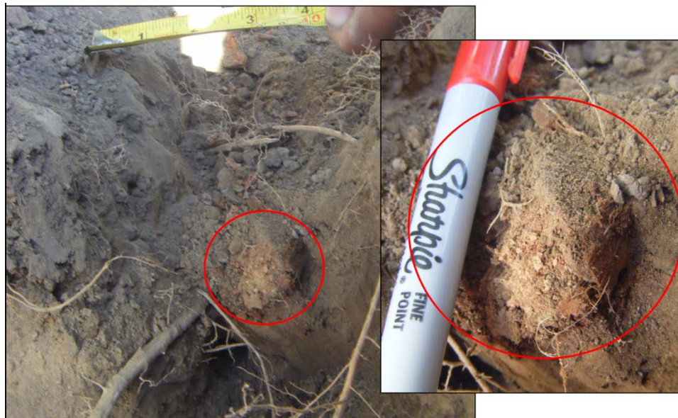
Figure 2-77. Close in view of decomposing root at Station 155. No gap was observable around this friable and highly decomposed root.
