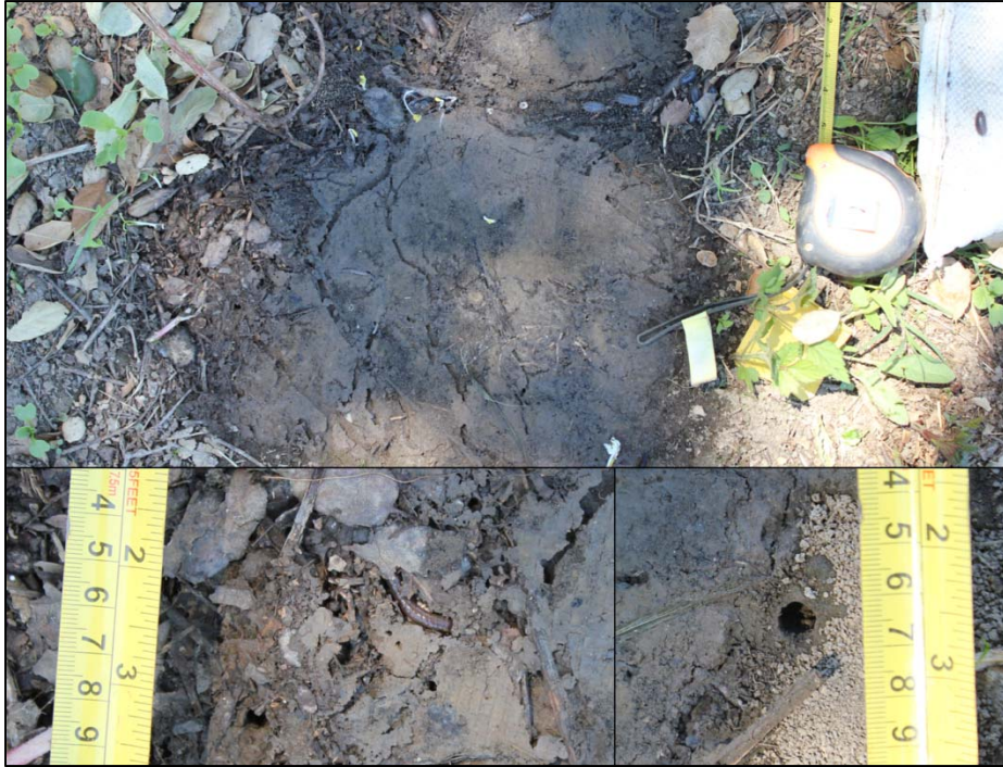
Figure 3-172. Station TT 57 to 59 seepage location upon lifting gravel bags. Worm traces were abundant and \frac{1}{4} inch diameter holes entering into the slope were occasional.
