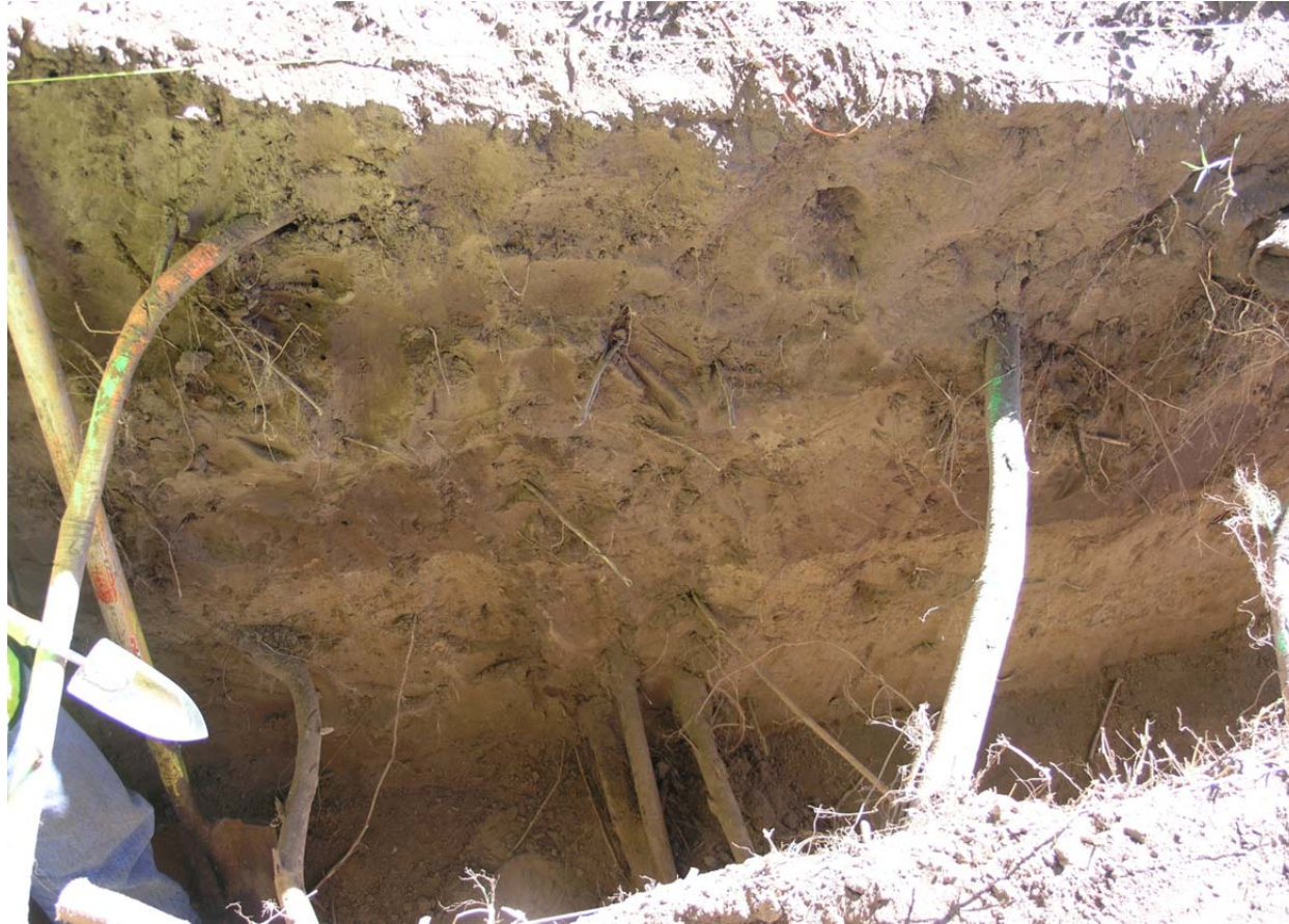
Figure 2C- 13. Stations 143 to 147 excavated to full depth and showing a cluster of decomposing and live roots as well as a 1.5 inch diameter pipe identified as a water line based on USACE documentation (USACE, 1999) as summarized in Appendix C.
