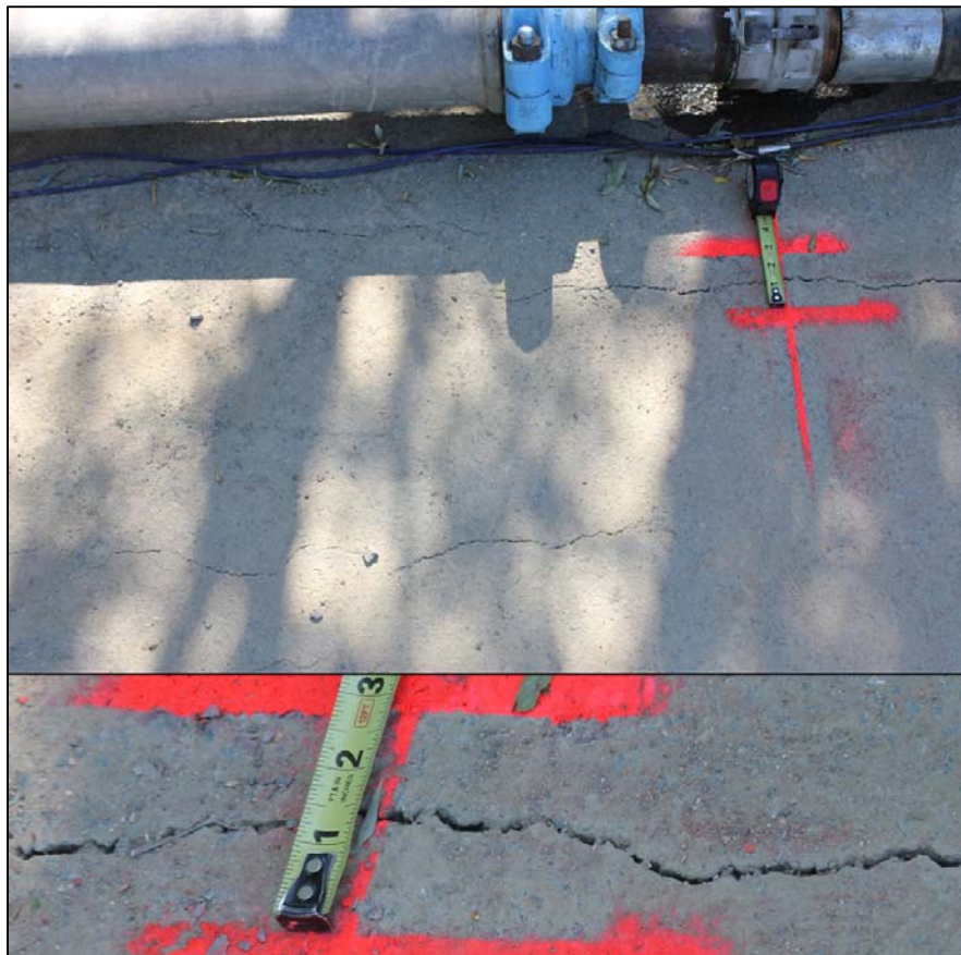
Figure 3-119. View of Stations TT 57 to 62 where cracking was observed in pavement 25.5 hours into the flow test. A monitor was installed at Station TT 58.5.
