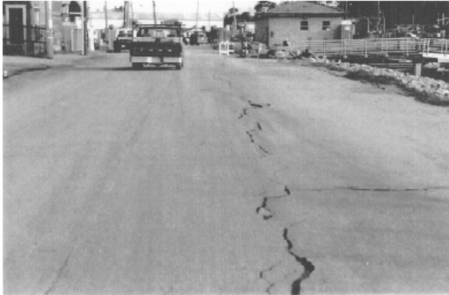
Figure 5-22. Cracking along Sandholdt Road (looking north just south of MBARI pier; from Boulanger et al. 1995).
