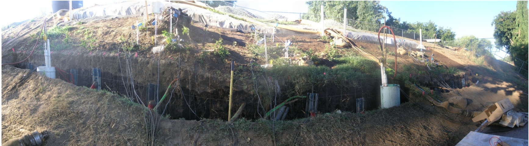
Figure 2-53. Wide angle view of saturation patterns at 67.9 hours into the flow test. The area below the stump has begun to saturate.
