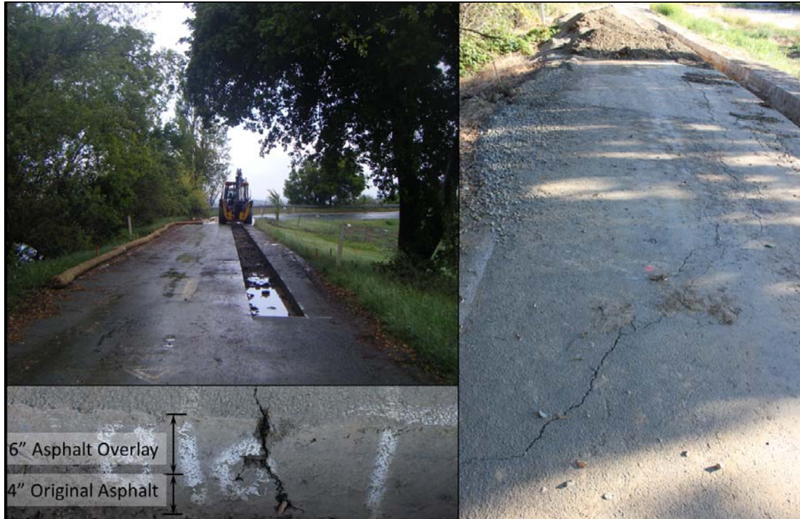
Figure 3-191. Pattern of pavement cracking (right) is similar to pattern of ponding in the pavement just following a rain event and prior to trench construction. Asphalt sections show evidence of a thick overlay, an indication of previous pavement distress.
