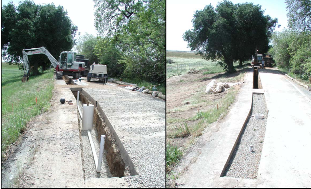
Figure 3-35. The control trench is partially filled with gravel, a manifold installed, and backfill with gravel is completed.
