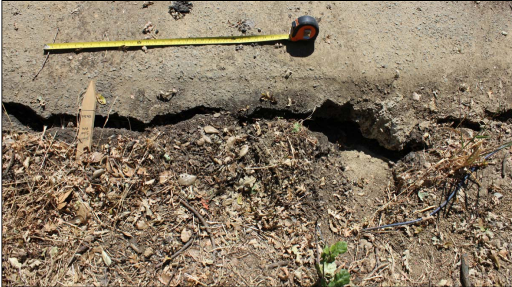
Figure 3-138. The grout of piezometer PB1 is intersected by the crack at the top of slope at the waterside oak.
