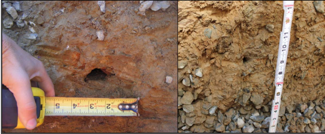
Figure 3-179. New burrow landside Station CT 10 at 18 inches deep (left) and new small burrow at landside CT 3 (right).
