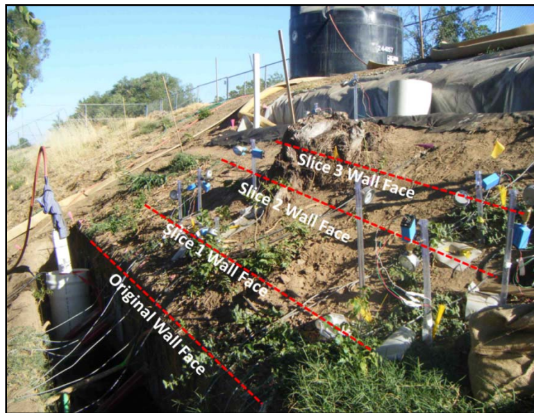
Figure 2-73. Excavation was completed around the stump in a series of vertical slices from Stations 138 to 153 as shown.
