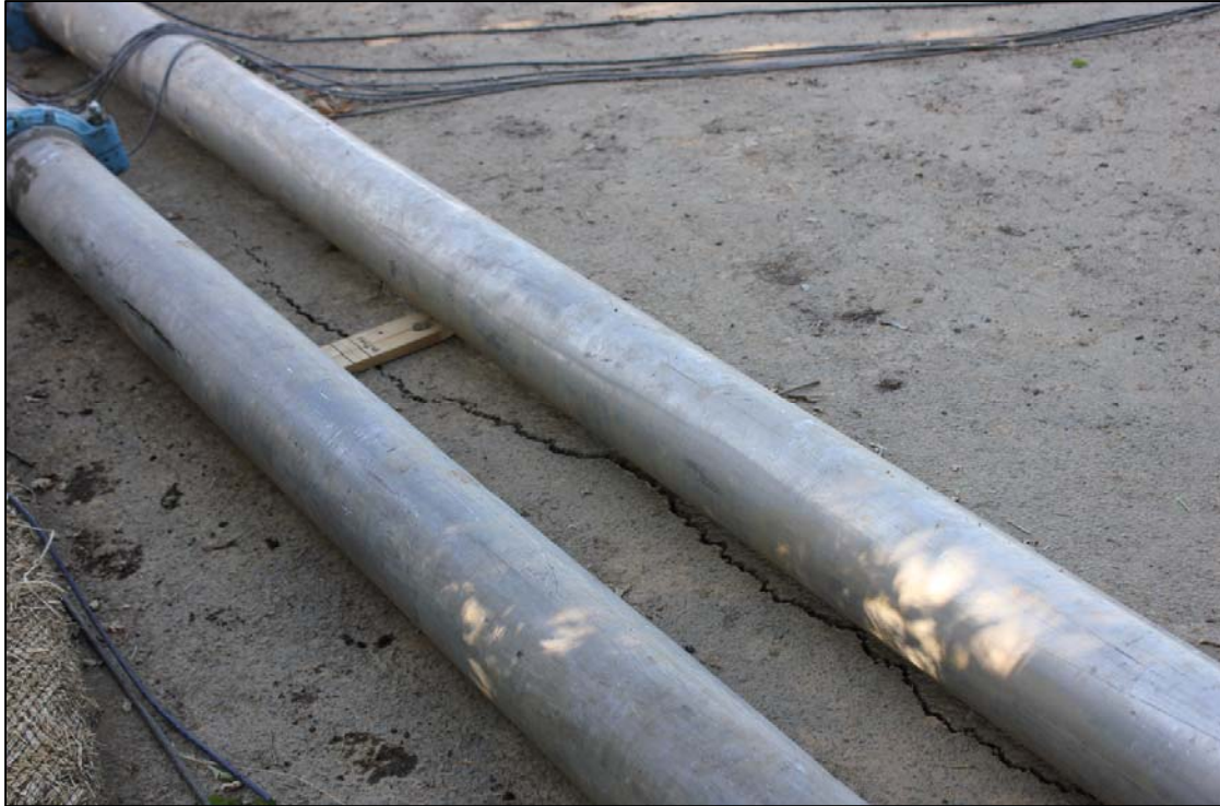
Figure 3-127. Crack discovered on 5/31/12. No additional movement was recorded on the monitoring device (Stations TT 40 to 52).
