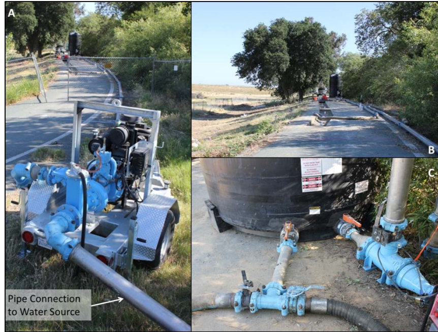
Figure 3-21. Pump and tank system (A and B). Image C shows valves used to control rate of flow into the trenches.
