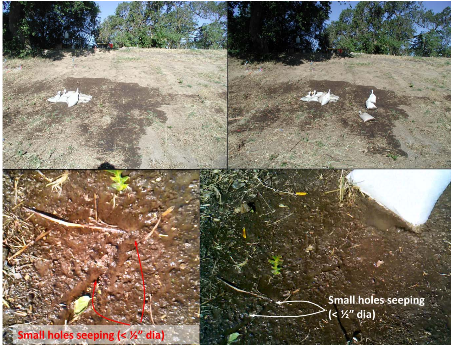
Figure 3-105. Time = 43 hours (8:45 am on 5/23/12). In the vicinity of Stations TT 45 to 60, seeps are observed to be flowing from tiny holes on the order of \frac{1}{4} to \frac{1}{2} inch in diameter (lower photos). Later exploration revealed worm burrows in these locations as discussed in subsequent sections.
