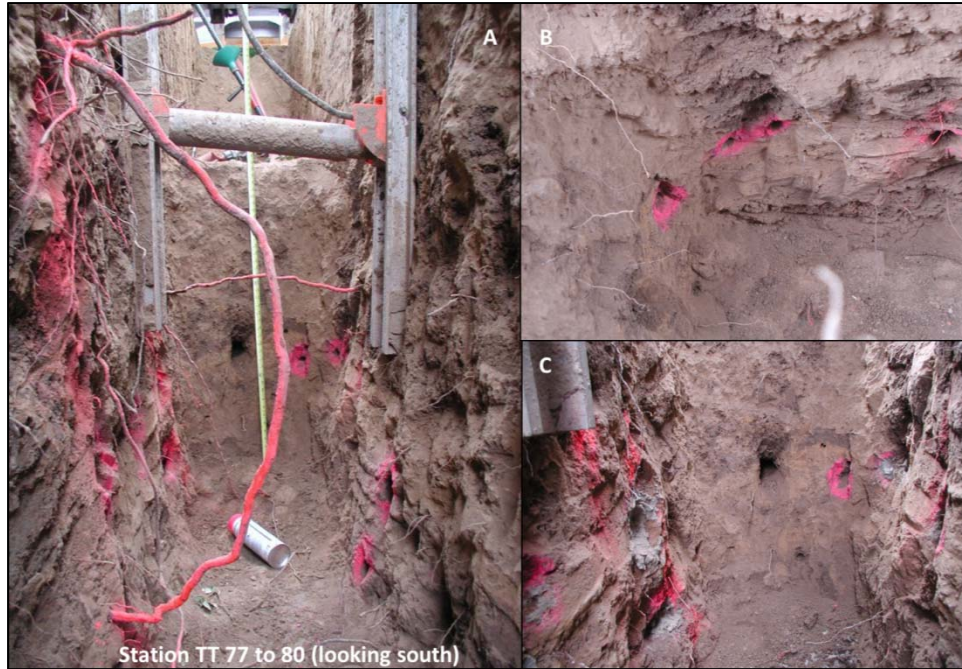
Figure 3-82. A) Overview of roots and burrowing activity (diameters from 1 to 3 inches) from Stations TT 77 to 80. B) View of 1 to 1 ½ in diameter holes at Station TT 81 waterside wall; C) View of 3 inch diameter burrow at Station TT 81.
