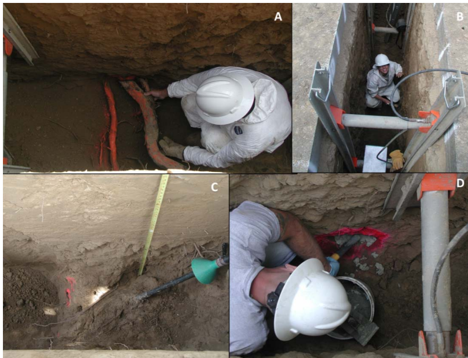
Figure 3-39. A) Large root at Station TT 17; B) Logging; C) Burrow found during air knife excavation; D) Burrow patched prior to flow test.
