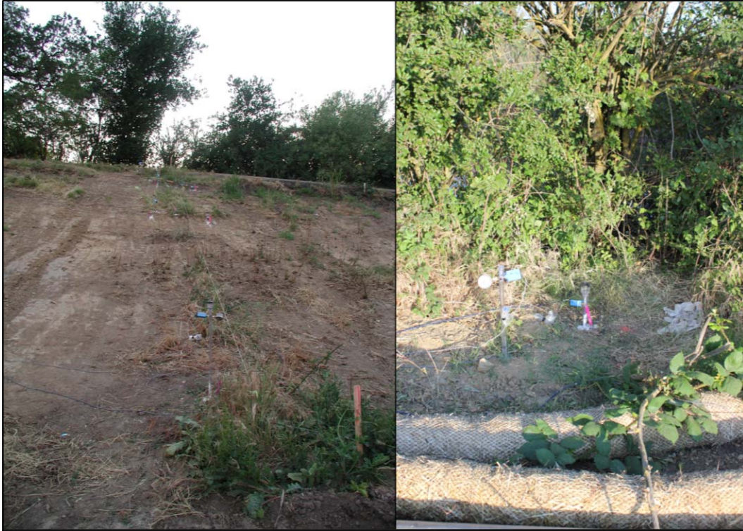
Figure 3-95. Instrument line C from the toe of slope looking west (left) and from the crest looking west at waterside instruments.
