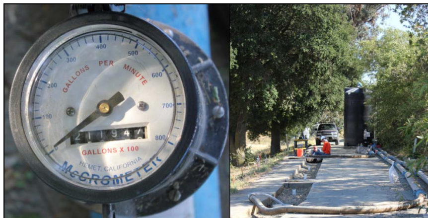
Figure 3-22. Typical flow meter (left) as installed on pipes flowing into and out of the 4900 gallon reservoir. Water delivery pipes and hoses are pictured to the right.
