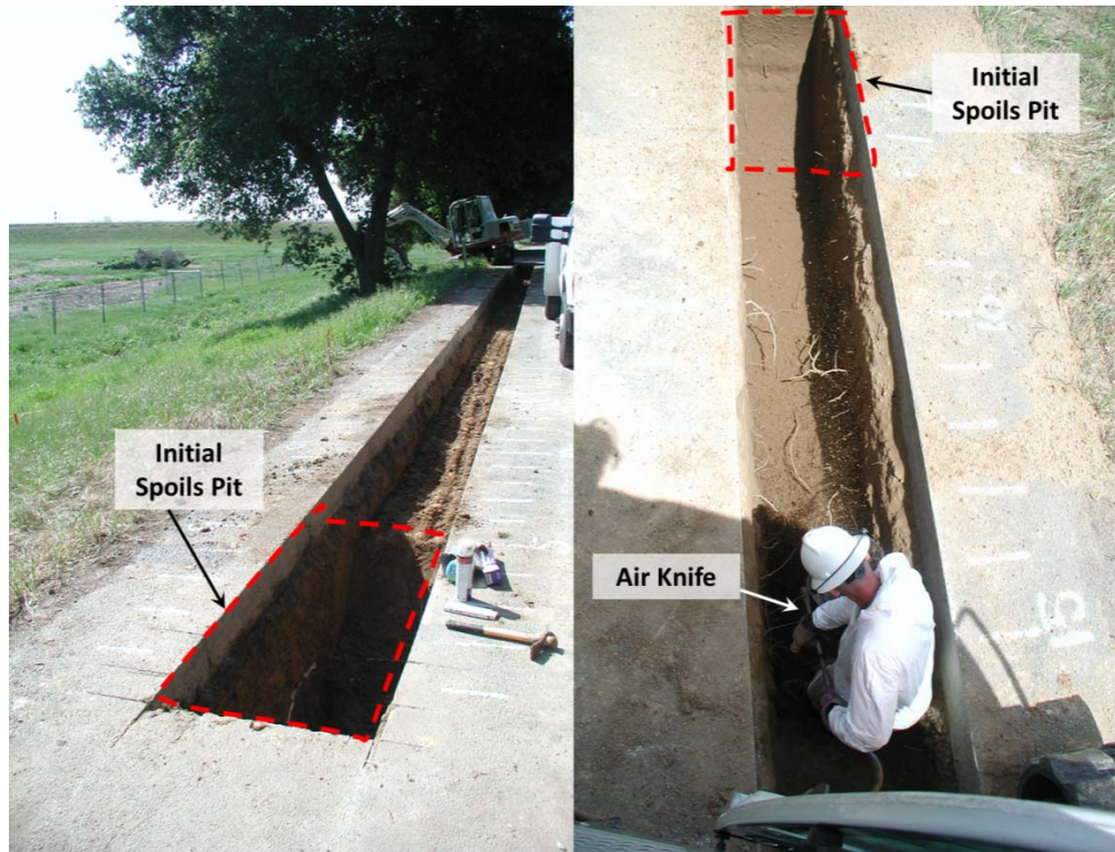
Figure 3-37. Initial spoils pit (left) and air knife operation revealing the upper 4 feet within Stations TT 5 to TT 15.
