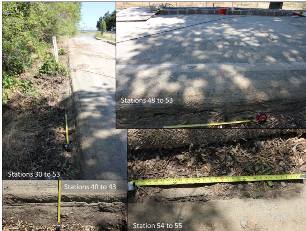
Figure 3-141. An older crack at Stations TT 30 to 55. Note dead plants rooted into the crack. Seepage at the waterside oak tree was the first location that moisture was observed coming out of the slope at approximately Station TT 20. The seep was first spotted at 10:40 pm on 5/21/12, 9 hours into the flow test, at the location shown on Figure 3-142. By 6 pm the following day, nearly 29
