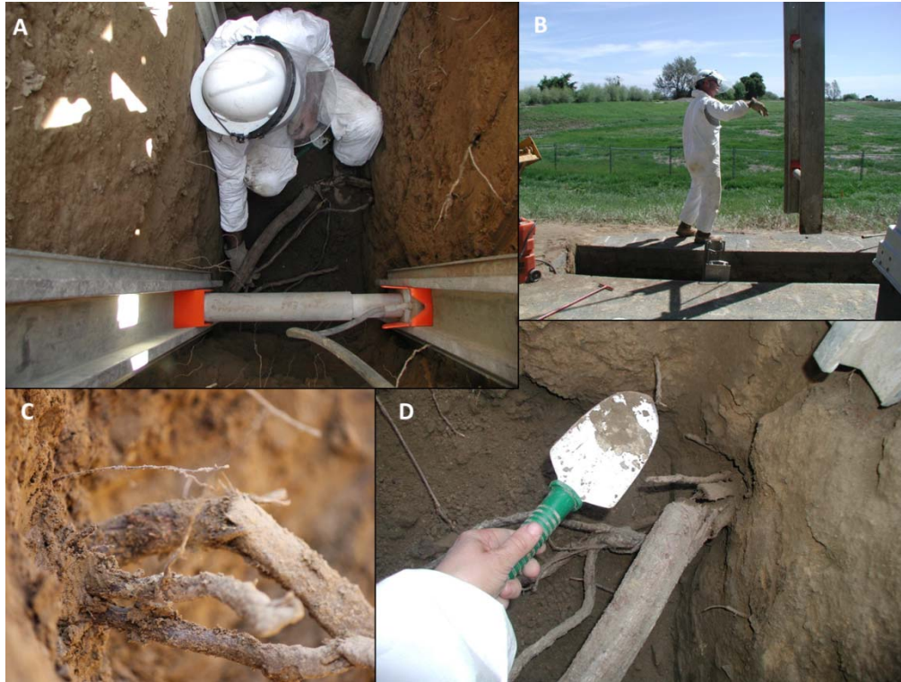
Figure 3-36. A) Root encountered during excavation of initial spoils pit at Station TT 0 to TT5; B) Trench is shored; C) and D) Roots damaged by excavation are carefully inspected at walls and found to be intact at connection to the wall.
