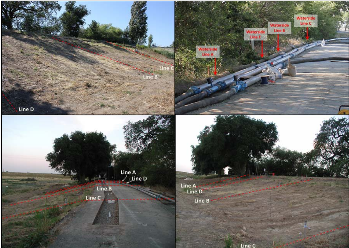
Figure 3-91. Photographic view of landside and waterside instrument line locations.
