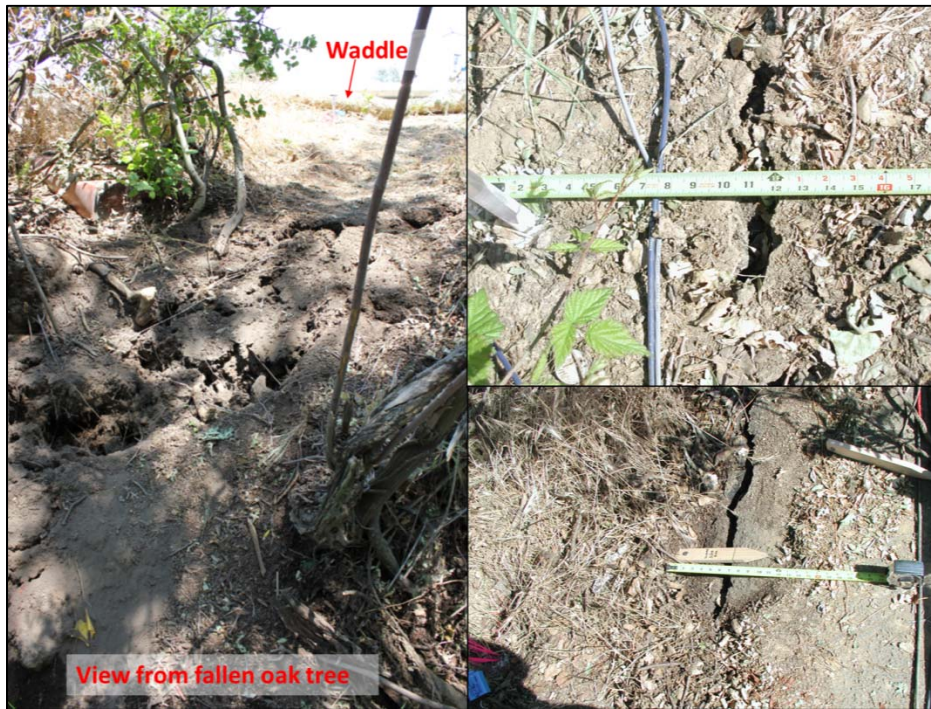
Figure 3-136. In the afternoon of 5/23, during a visit from Dr. Les Harder of HDR, a fresh crack was revealed along the top of slope, previously concealed by leaves and an erosion control wattle.
