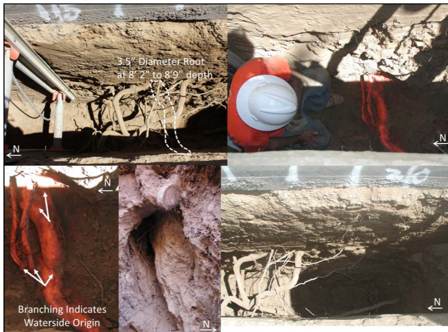
Figure 3-67. Station TT 15 to 20. Excavation extended below 8 feet to remove a 3.5 inch diameter root for constructability concerns (upper right, lower left). Void space was found in the soils at Station TT17 waterside (bottom center).
