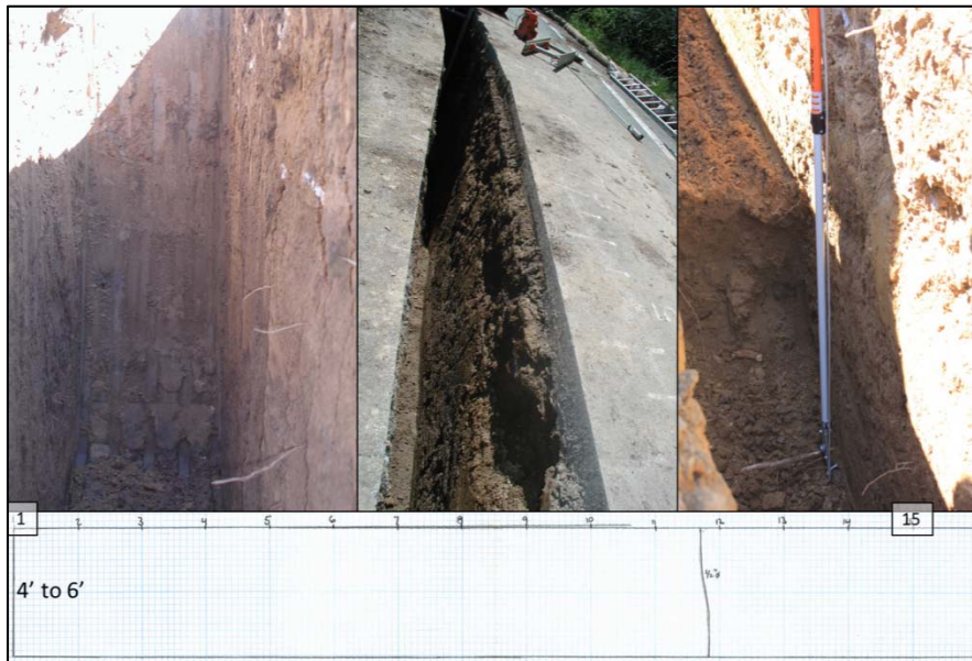
Figure 3-51. A single ½ inch diameter oak root is found and cut when excavating to full depth of 8 feet within the control trench Stations CT 1 to 15.
