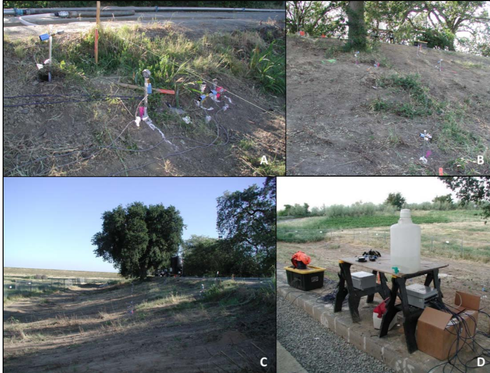
Figure 3-27. Instruments (photos A through C), once installed, are wired into readout boxes (D) for continuous readings during the flow test.
