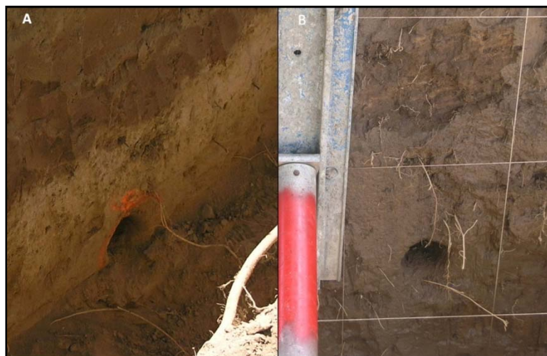
Figure 2-59. Squirrel burrow extending at least 18 inches into the uphill wall of the lower trench at A) the time of trench construction and B) 50 hours into the flow test. No free water flows until a seep upon saturation at 125 hours (See Table 2-2)
