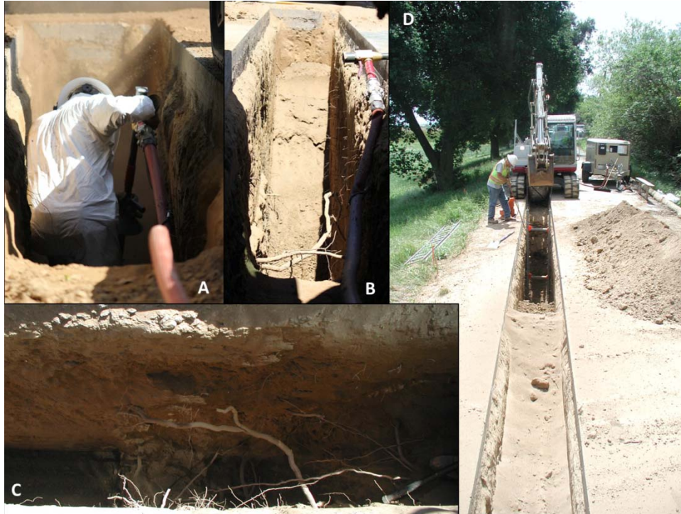
Figure 3-38. A) Air knife operator stands in 4 foot deep trench excavating to 8 feet; B) and C) New roots revealed as air knife spoils are blown in the previously logged segment; C) Spoils are used to stabilize previously excavated sections as new excavation proceeds.
