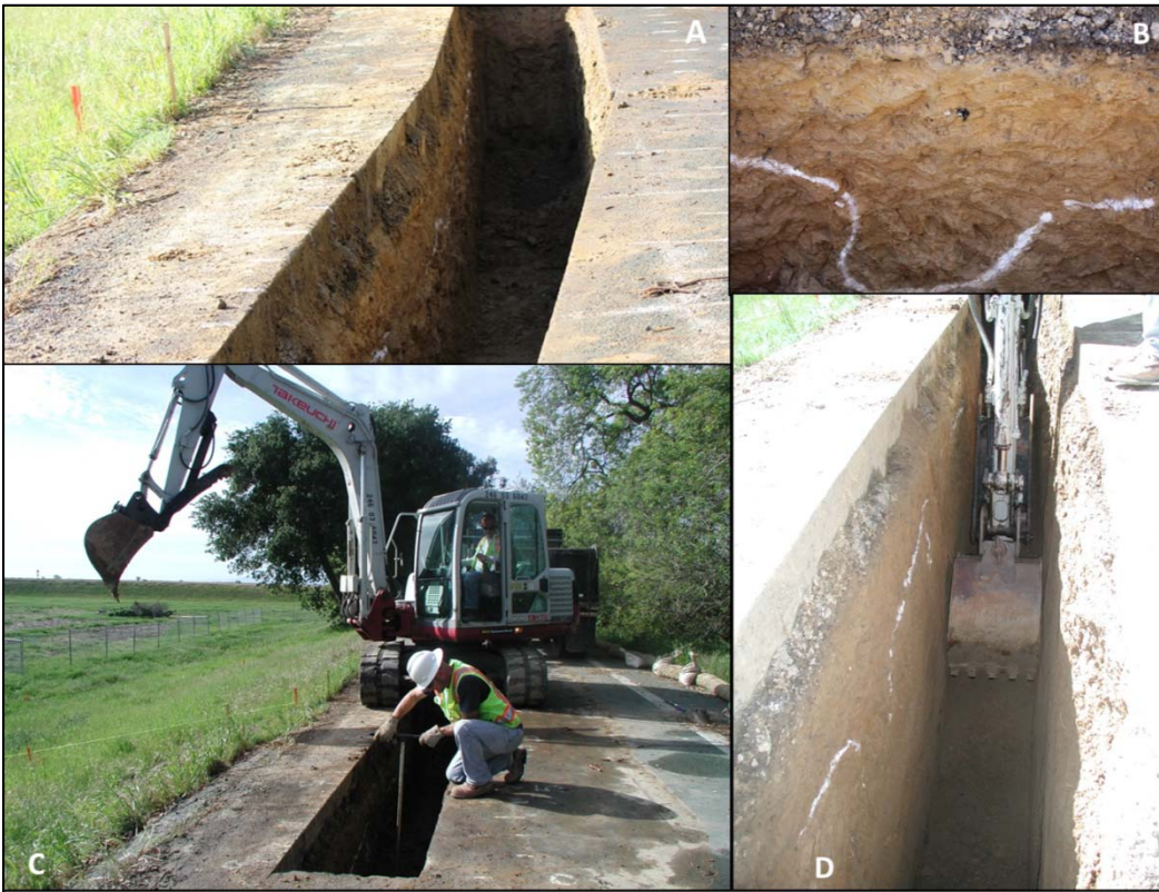
Figure 3-33. A) The control trench excavated to 4 foot depth; B) Walls are logged; C) Walls are sampled ahead between 4 and 8 feet; D) Excavation of small segments proceeds to 8 feet.
