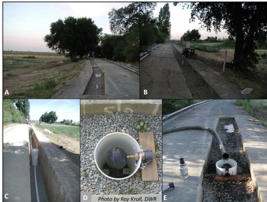
Figure 3-23. Gravel filled A) Control trench and B) Tree trench. The water delivery manifold (photo C), the constant head mechanical float (photo D), and the delivery hoses (photo E) are shown.
