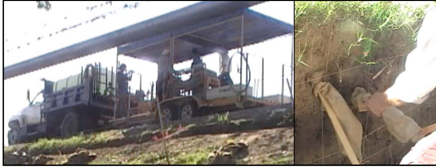
Figure 2-74. ARFCD grout plant and trailer combination is shown (left). To the right, burrows are plugged with burlap sacks using a rod leveraged against the ground in order to prevent loss of grout.
