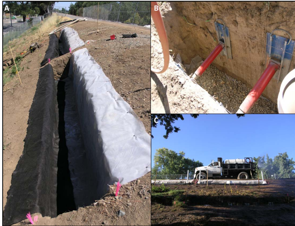
Figure 2-38. Trench preparation prior to commencement of flow. A) Upper trenches lined with plastic sheeting (uphill and base walls) and permeable fabric (downhill wall); B) shored lower trench lined with plastic sheeting and gravel (base); C) water truck moistens site to prevent cracking prior to flow test.
