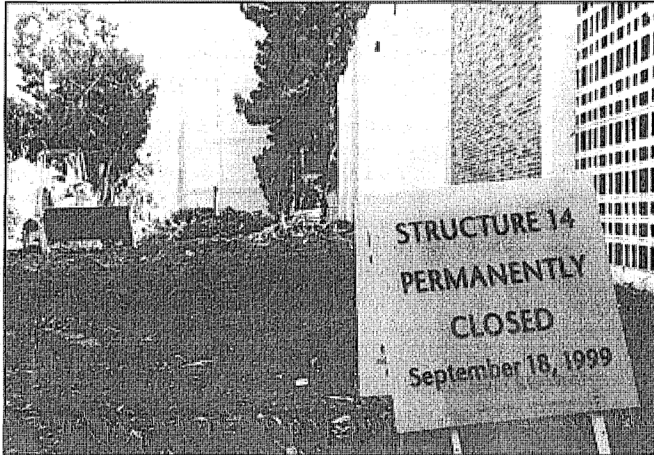
Bulldozers will soon scoop up precious parking space when Lot 14 is demolished
