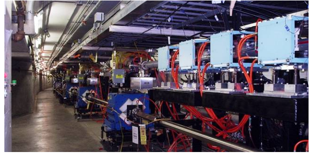
Figure 4. Chicane dipole magnets (Right) installed in the LER (upper beam pipe) for electron cloud tests.
