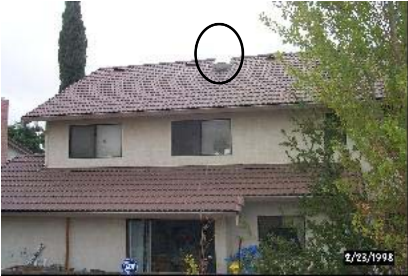
Figure 10. Installed roof mounted economizer vent.
