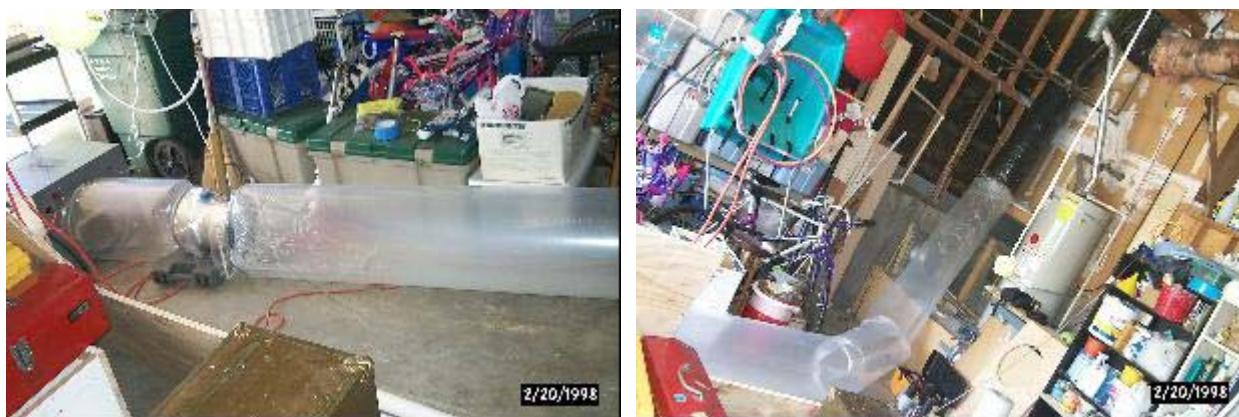
Figure 17. Aerosol apparatus for duct sealing in garage.
