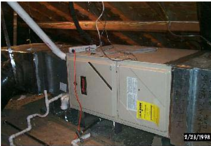
Figure 7(a). New cooling and heating equipment on attic floor [right to left: return plenum, air filter, air handler, furnace, cooling coil and supply plenum].
