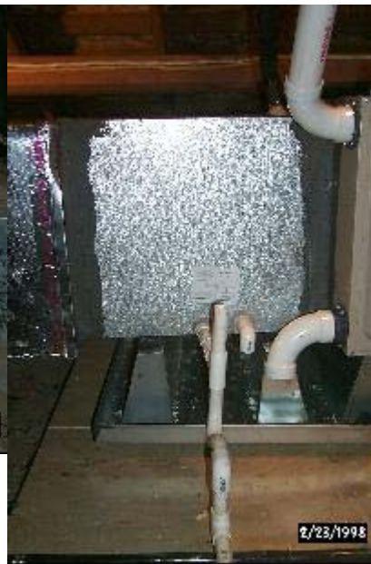
Figure 7(b). New cooling coil with condensate drains and top of furnace with combustion air intake and exhaust.
