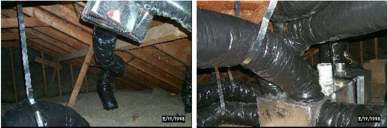
Figure 12. Initial installation of ductwork hanging from ceiling of attic [right shows smooth bend out of plenum].
