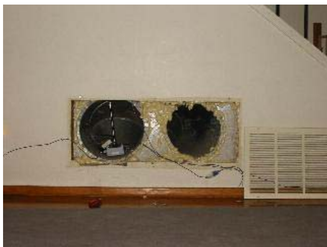
Figure 16. Duct sealing of downstairs return using foam. [the sensor that is visible is a relative humidity sensor, there is also a temperature sensor in the duct].
