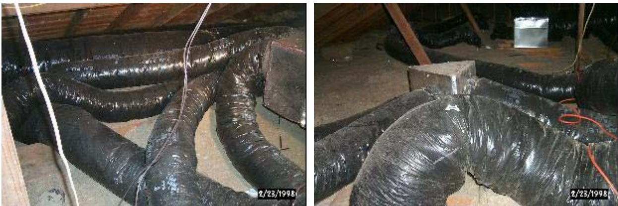
Figure 14. Second and final installed retrofit of ductwork after being moved to attic floor and before adding insulation showing tight bends.
