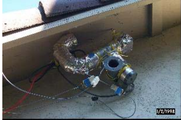
Photo B.2. Outdoor air aspirated temperature and relative humidity sensors located under roof eave.
