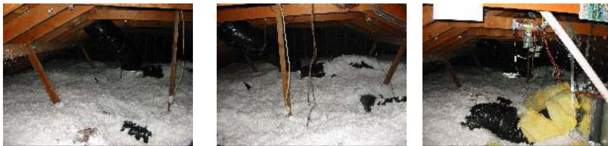
Figure 15. Attic floor with flexible ducts and additional blown-in insulation over ducts. The yellow material is fiberglass wrap insulation.
