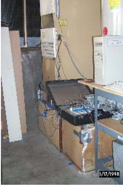
Photo B1. Data acquisition equipment in garage with existing furnace in background.
