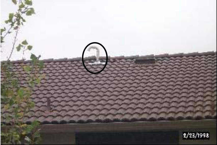
Figure 9. Installed roof mounted furnace flue pipe.
