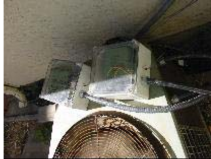
Photo B.5. AC condensing unit power meters, one each for the compressor and condenser fan motors.
