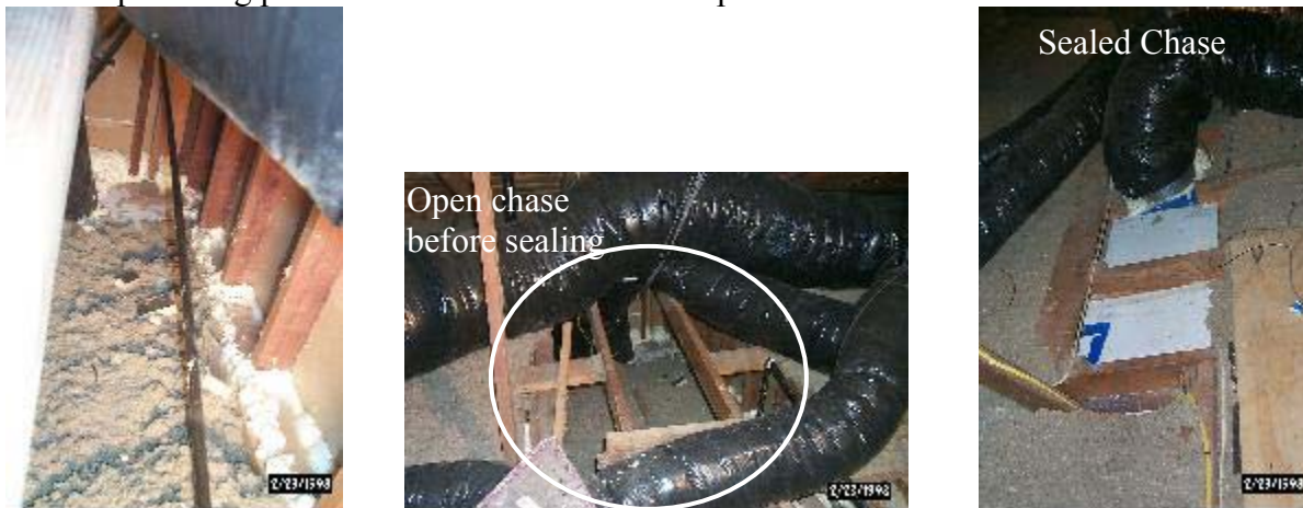
Figure 6. Sealing cavities connecting the house to the attic. Foam is a useful sealing tool for small holes and cracks at building component intersections (left). Duct board insulation can be used to block off large open areas (center and right)
