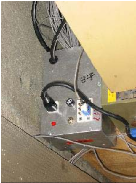
Photo B.6. Air handler power meter located in garage.
