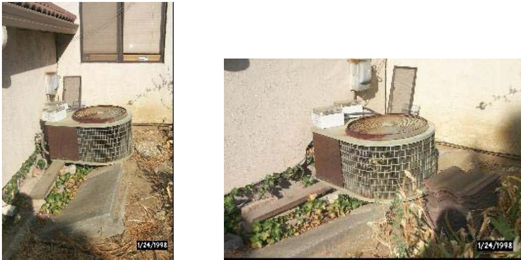
Figure 4. Existing AC condensing unit outside near rear of garage showing poor condition of unit [heavily corroded sheet metal fasteners and significant dirt/dust accumulation blocking flow into coil] and subsided slab [stressed refrigerant tubing and subsequent leakage of refrigerant].
