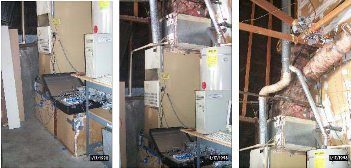
Figure 3. Existing HVAC equipment in garage [left to right: return plenum, air handler, furnace, cooling coil and supply ducts].
