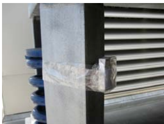
Figure 4.9 Location of exterior rooftop temperature sensor.
