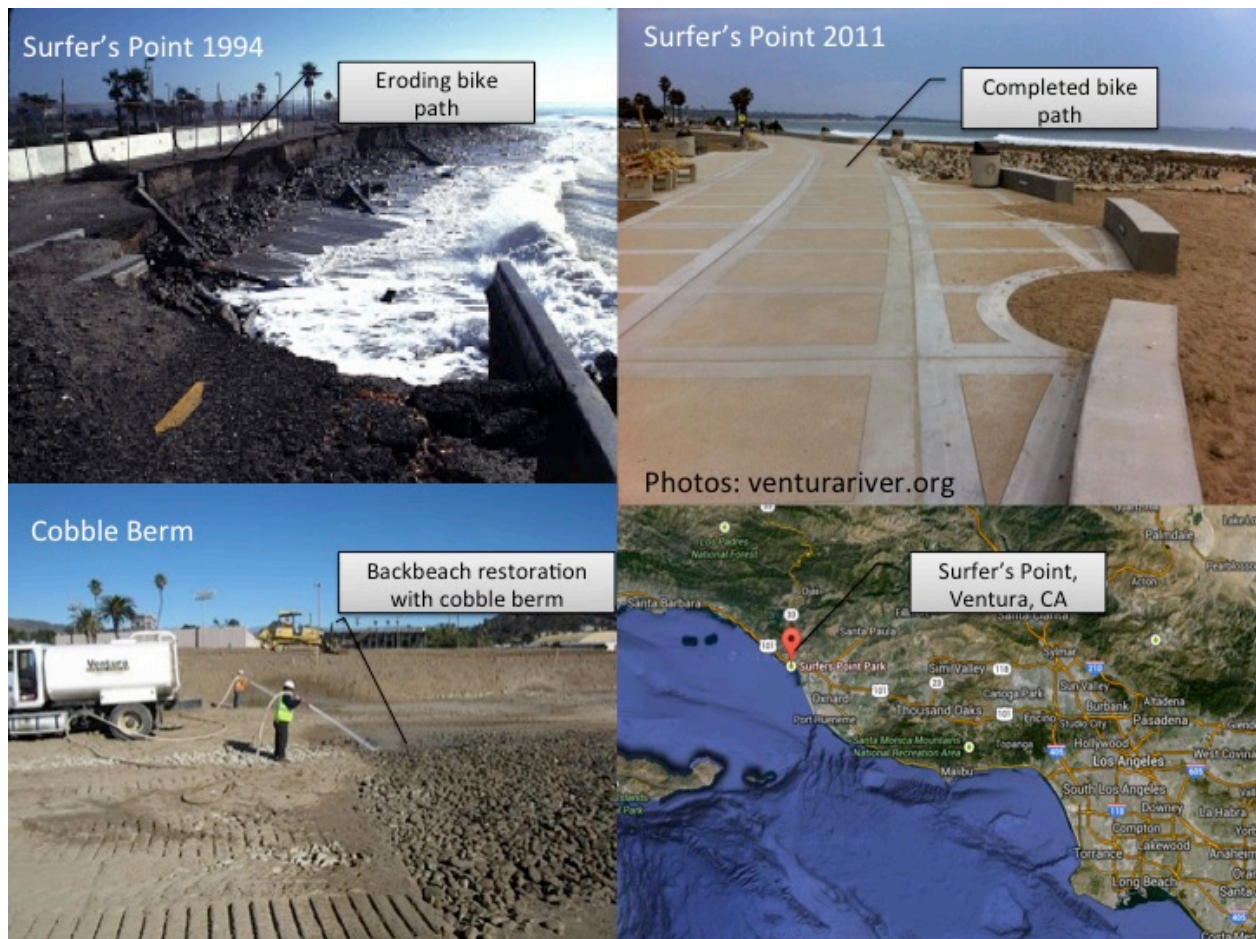
Fig. 3 Map of Surfer's Point location and photos of managed retreat project. Top left: original bike path and erosion damage, bottom left: construction of cobble berm, top right: completed bike path phase 1 construction, bottom right: map of California with Surfer's Point labeled
