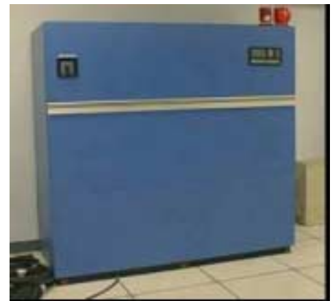
Figure 12 Typical CRAC unit
