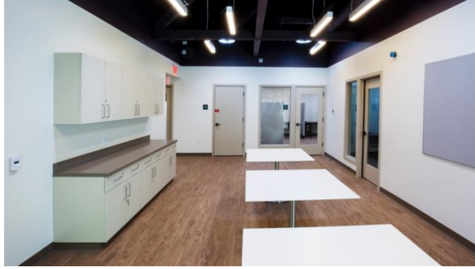
Figure 14: Interior Breakroom with Installed Tubular Daylighting Devices
