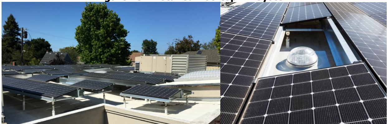
Figure 13: Installed Rooftop PV System
