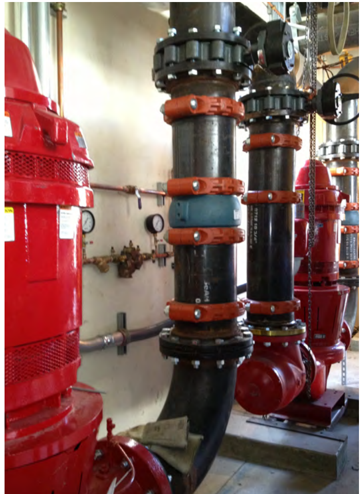
Central plant chilled water pumps and pipes prior to insulation.
