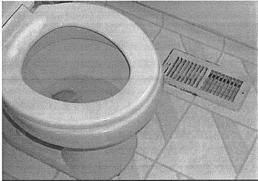
Figure A-4. Example of a register that is hard to access. The only way to measure flow at a register like this is by using a bag with a flexible wire coat hanger around its entry that can be formed into a shape to fit in the available space
