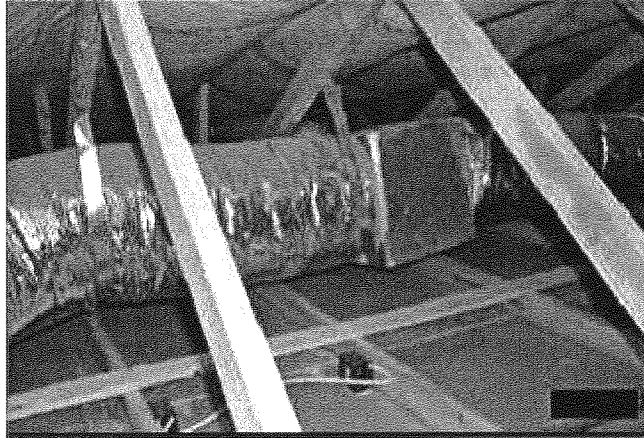
Illustration of an unvented attic. The insulation has been moved from the attic floor to the pitched roof surfaces and all the attic vents have been sealed. Because the attic is now inside conditioned space – the ducts losses are very small.
