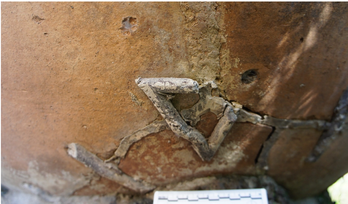
Fig. 4.30. Partially preserved lead alloy triangular clamp (and hybrid clamp and mortise and tenon) repair (II.8.6 n. 1), Pompeii.
