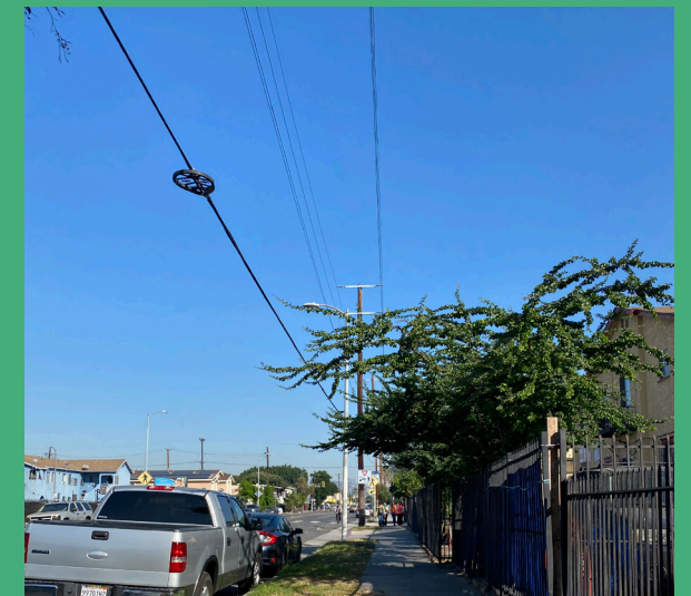
Figure 4. Overhead power lines
