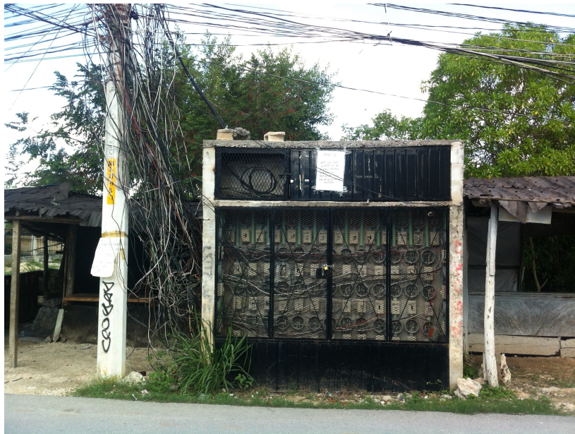
Figure 4.3: Electrical transformer hooked up to electrical lines extending from the main highway. Since there are no individual meters on the transformer, everyone connected to the transformer must split the electrical bill evenly.
