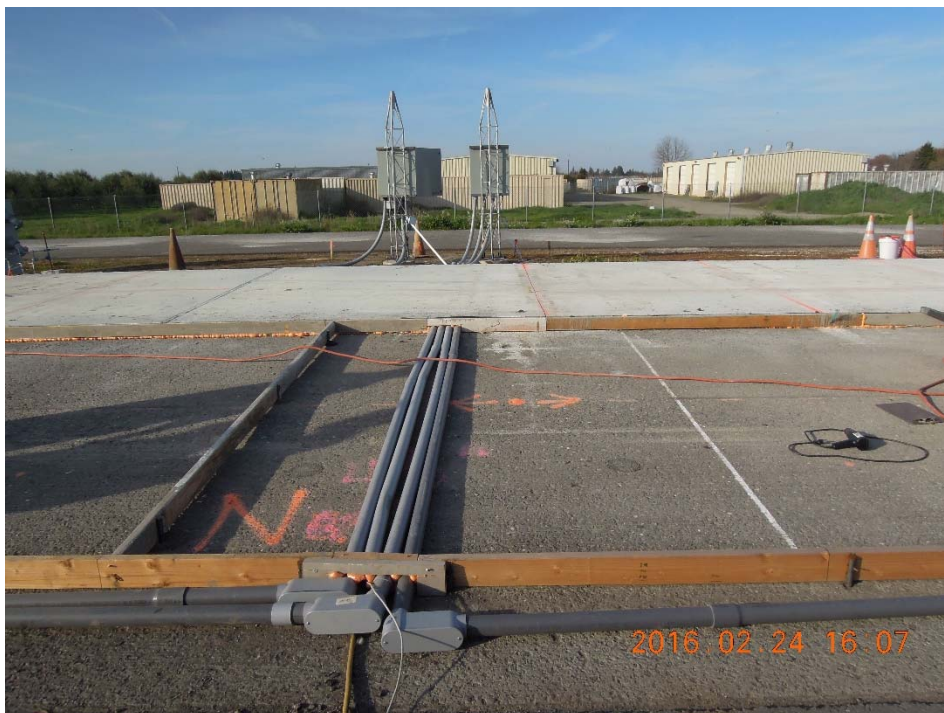
Figure A.26: Pipes running instrument wires across the pavement structure.
