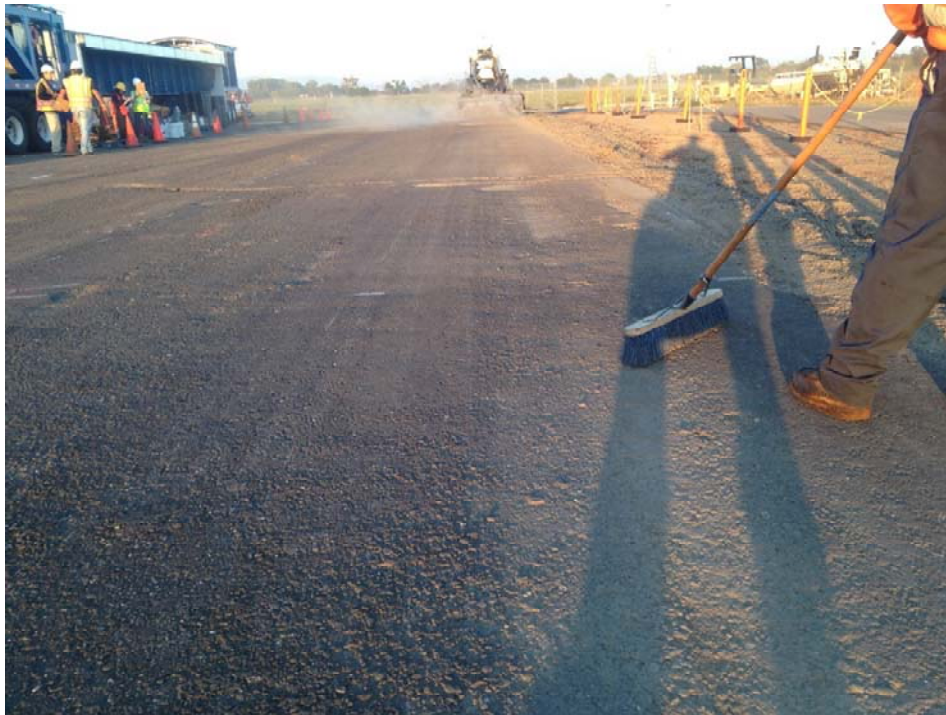
Figure A.1: Full-depth reclamation (FDR) surface cleaning and preparation prior to placement of new HMA.
