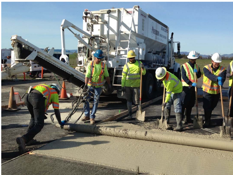
Figure A.54: Volumetric mixer and CSA concrete consolidation with hand-operated roller screen.
