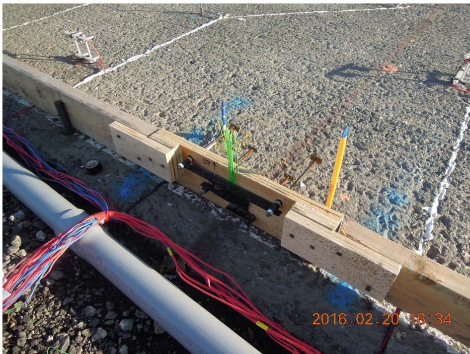
Figure A.18: Close-up of the anchoring rods for the JDMD targets and rod of IOMD protected by yellow straw.
