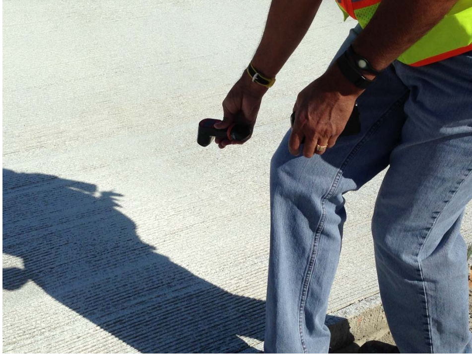
Figure A.71: Tracking the surface temperature on the CSA section.
