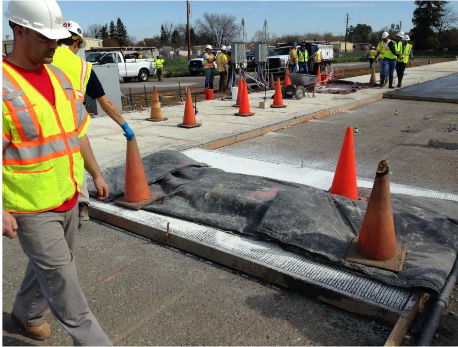
Figure A.93: Beams on top of pavement slab, under insulation blanket (California Test 524).
