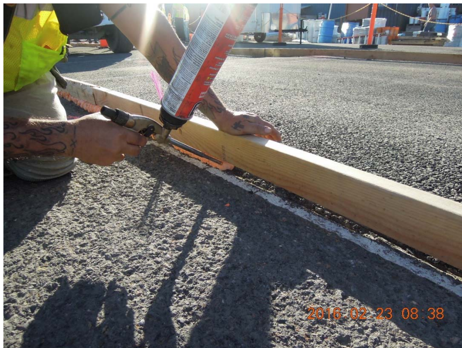
Figure A.48: Filling the gap between asphalt and form work with foam.
