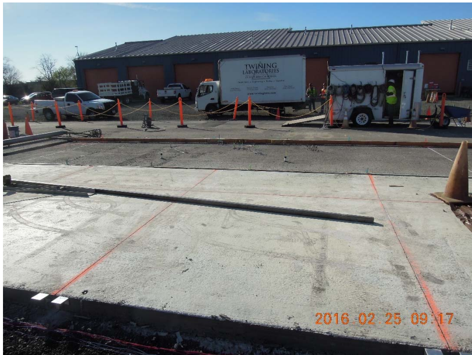
Figure A.78: Lane 1 (first plane) and Lane 2 (beyond Lane 1) ready to be paved.
