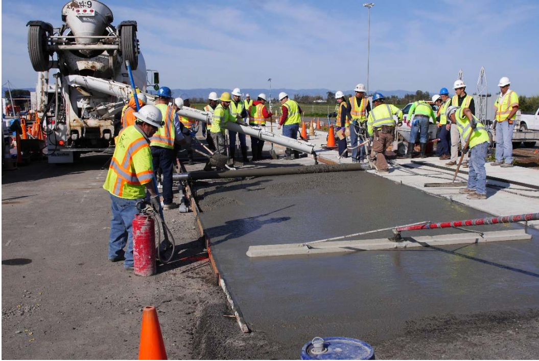
Figure A.97: Concrete pouring (discharge chute), consolidation (roller screed), and finishing (bull float).
