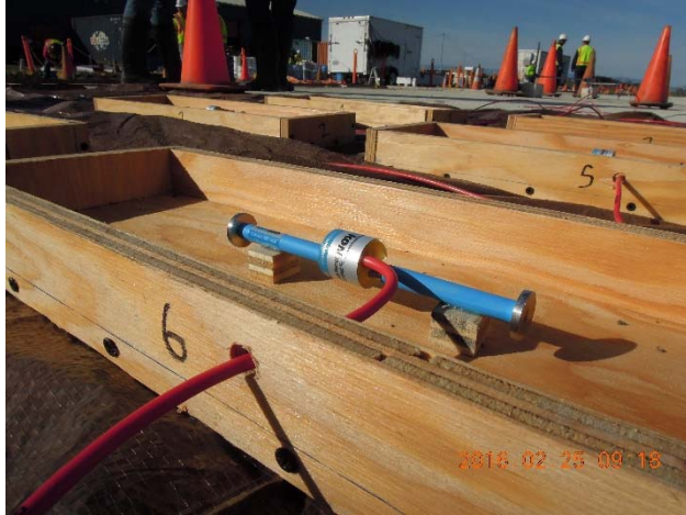
VWSG inside the mold
