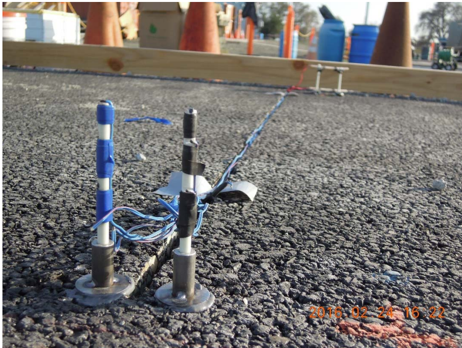
Figure A.28: Close-up of two sets of thermocouples.
