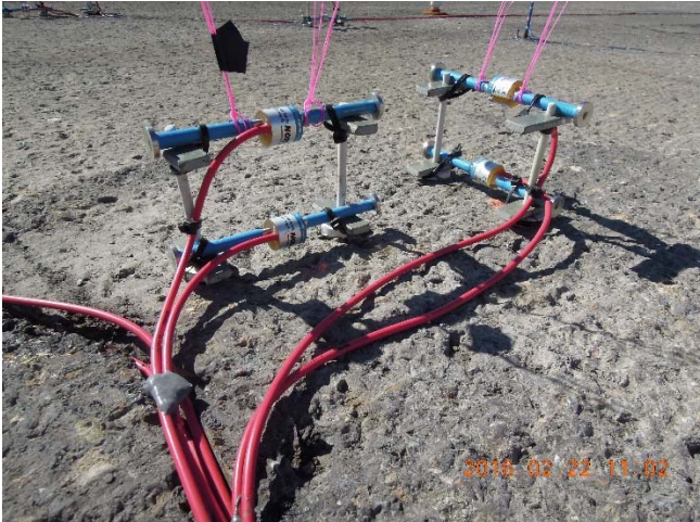
Static strain gages (two longitudinal, two transverse) Note: the pink threads will mark the exact location of the VWSGs after overlay paving. The exact location of the gages was required for forensic coring.
