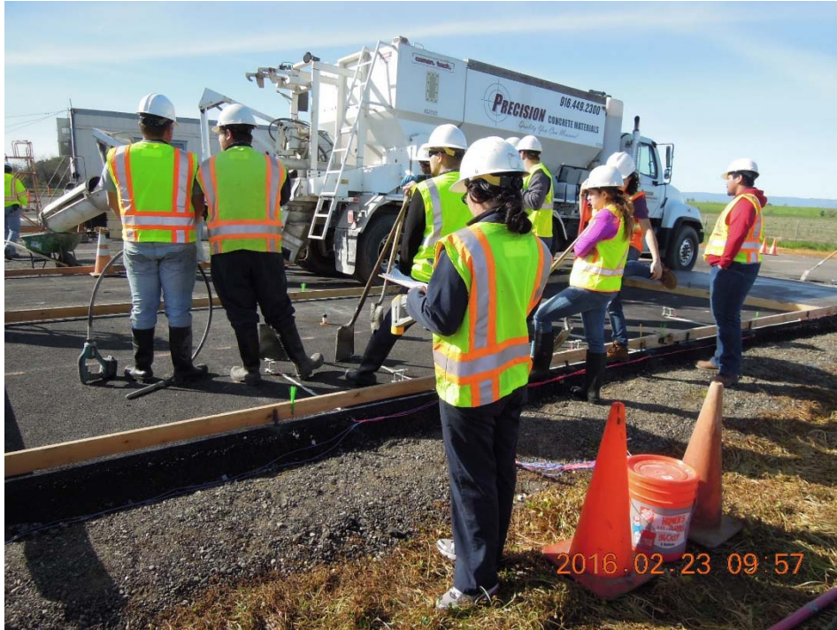
Figure A.53: Volumetric mixer ready to mix and pour the CSA concrete.
