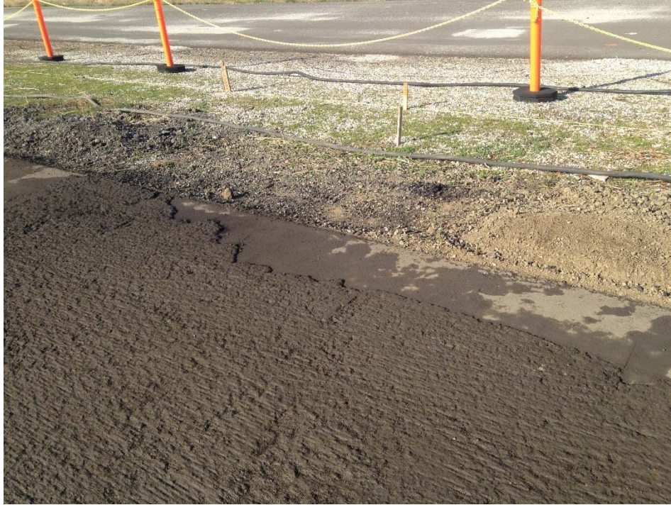
Figure A.11: Old asphalt surface after milling (note debonding between the two asphalt lifts).
