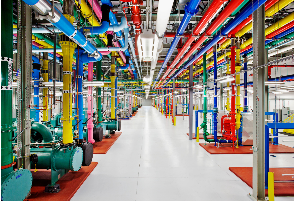
Figure 2. A central cooling plant at Google data center in Douglas County, Georgia. Copyright © 2013 Connie Zhou. Reprinted by permission.
