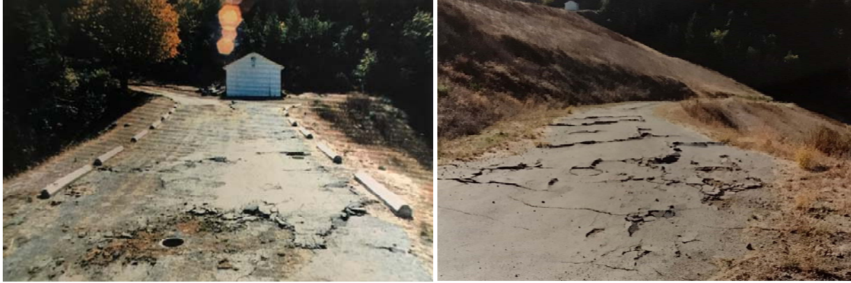
Figure 5. Photographs of cracking after Loma Prieta earthquake: (a) longitudinal and transverse cracking on the dam crest near the left abutment, (b) cracking along access road on the lower portion of the downstream face (California Division of Safety of Dams files 1989)
