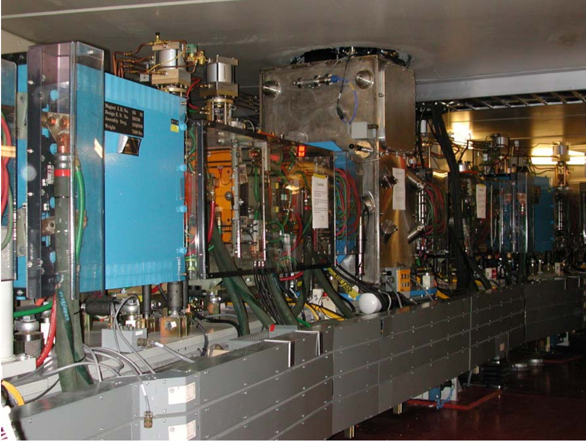
Figure 4. Superconducting dipole magnet (large silver-colored magnet in center) in the Advanced Light Source storage ring. Since the August 2001 installation of the superbends in three of the 12 sectors, which has extended the ALS spectral range well into the hard x-ray spectral region, several new beamlines for protein crystallography have become operational. Additional beamlines are under construction or planned for crystallography, tomography, and high-pressure research (diffraction and spectroscopy).
