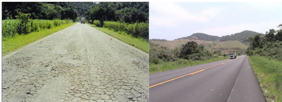
Figure 2.12: Highway RJ-122 pavement in Brazil before and after overlay placement with an ARFC surface.
