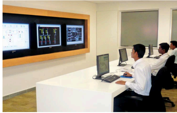
FIGURE 34: Building facility technicians monitoring the BMS at the Suzlon One Earth, Pune campus. (Picture: Synefra 13 )
