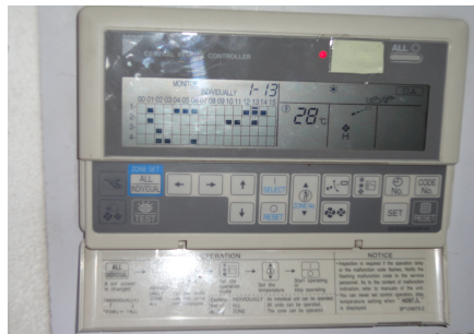
FIGURE 11: Air conditioning controls at Sears Holdings, Pune, offices. Thermostats are set at 24°C. If occupants leave their office for a few hours, they reset their individual thermostats to 28°C in order to save energy. (Photo: Facilities Team, Sears Holdings India)
