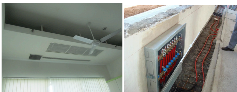
FIGURE 14: (Left) Air distribution from the DOAS through vents; (Right) A manifold at the perimeter workstations controls the tube water temperature. (Photo: Infosys Green Initiatives Team)
