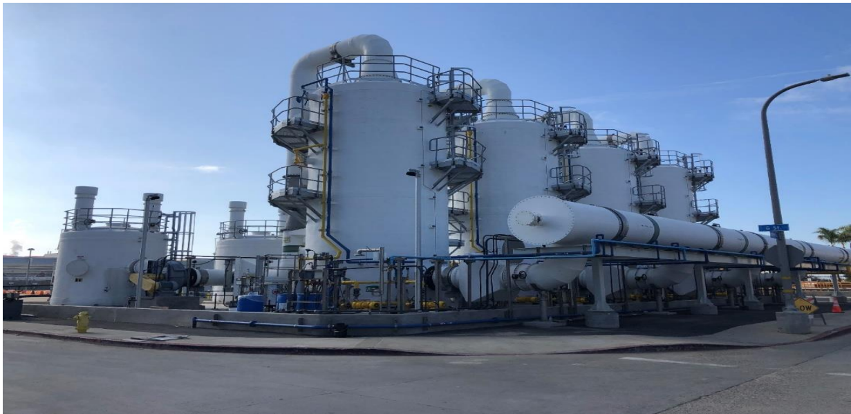
Figure 15. Hyperion Water Reclamation Plant (HWRP) Intermediate Pumping Station Odor Control BioTrickling Filter with Four BTFs & Four Carbon Scrubber Tanks in City of LA.
