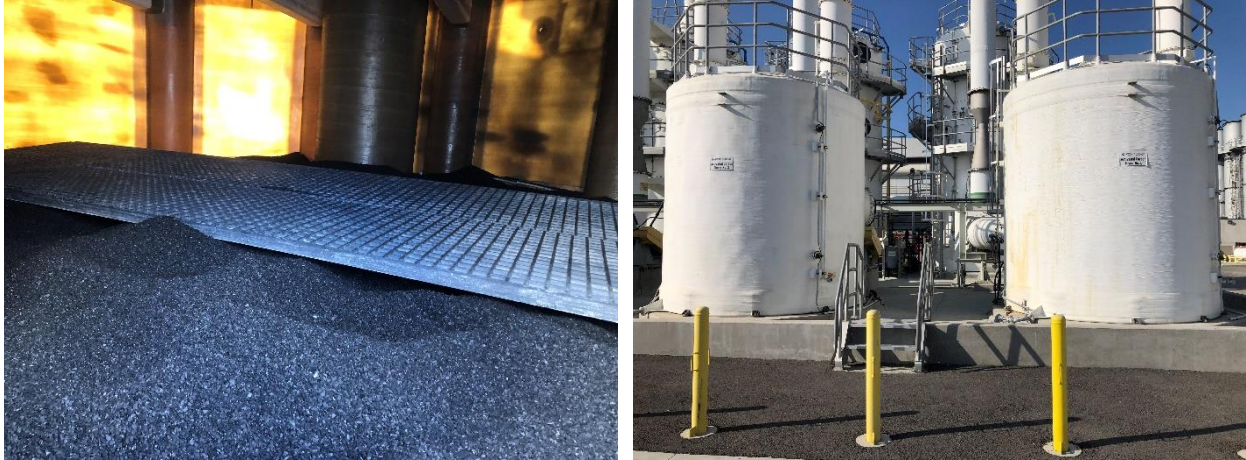
Figure 14. HWRP IPS Odor Control Pictures of Inside and Outside the Carbon Adsorbers Towers.
