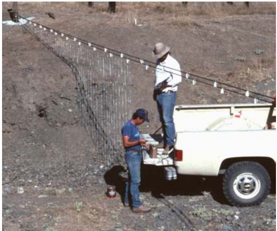
Center ag technicians Dana Edson and Steve Fernandes install fence to protect Parsons Creek riparian zone, October 1992
