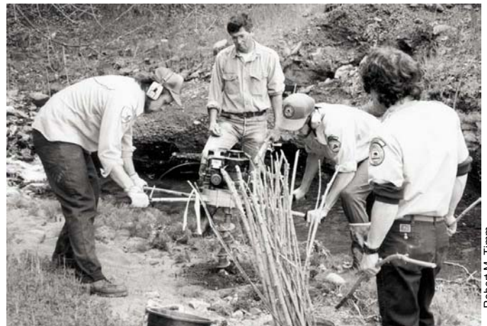
Bob Keiffer (second from left) coordinates planting of riparian vegetation along Parsons Creek, aided by Calif. Conservation Corps personnel, Spring 1993
