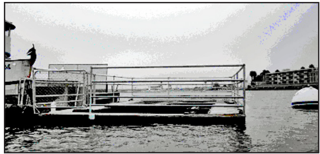
Figure 5. Bait receiver in Redondo Beach, California after installation of fence. Shown here is PVC piping on top of the galvanized aluminum fencing bolted to the dock with standposts, with 2 access gates for personnel and patrons to access the bait.
