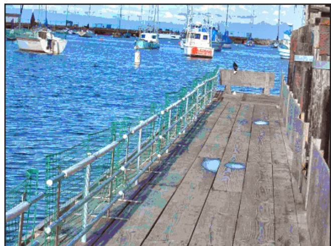
Figure 6. Dock in Monterey Bay, California after installation of fence. Shown here is PVC piping on top of aluminum fencing bolted to the dock, with green construction fencing on the dock side. At the end of the dock is a removable plywood structure to permit the release of a trapped animal, should it gain access to the dock.
