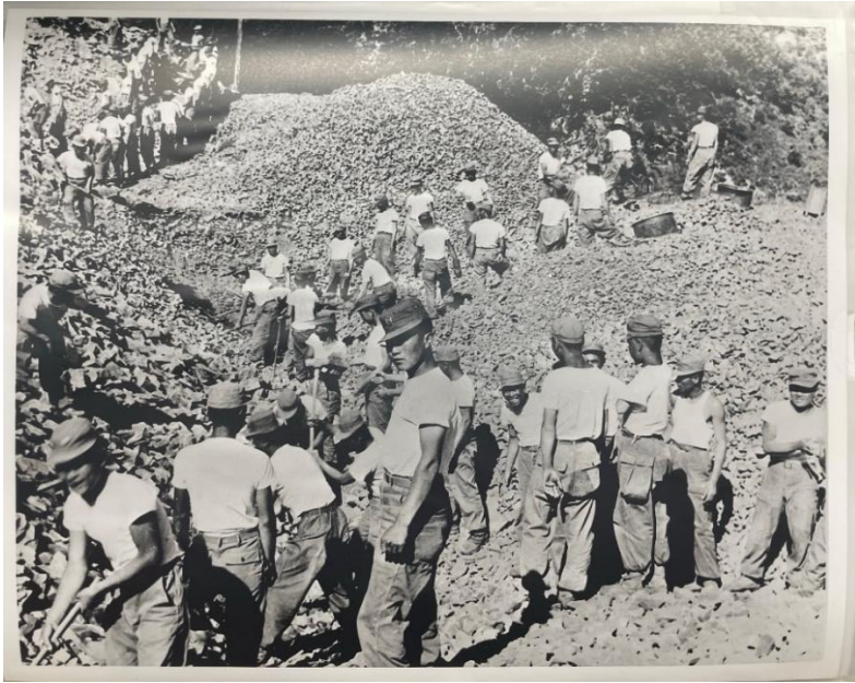
Figure 3.5. Soldiers carrying rocks from the Yeongam Line construction site with no heavy equipment on site. Circa. 1954. “Folder: Korean National Railway, Construction, Technical Assistance - Korea, 1955-1956.” Collection of Utah Construction Co./Utah International, Series 120/3/2 1-2.7, MS 100, Box 94. Weber State University Library.
