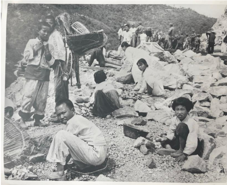
Figure 3.4. Local children mobilized to the Yeongam Line construction site. Top left is a child carrying an “A-frame.” Circa. 1954. Folder: “Korean National Railway, Construction, Technical Assistance - Korea, 1955-1956.” Collection of Utah Construction Co./Utah International, Series 120/3/2 1-2.7, MS 100, Box 94. Weber State University Library.
