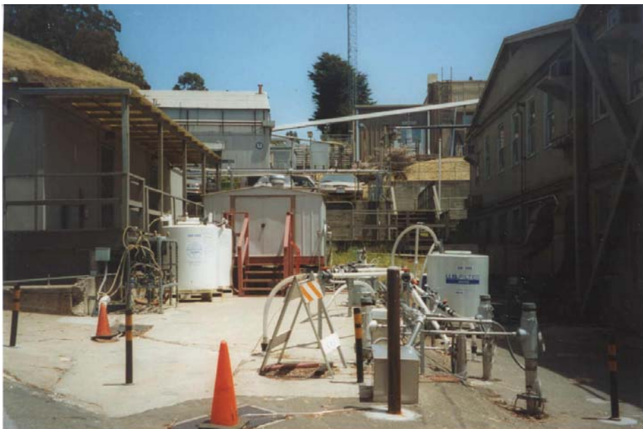
Pump and treat equipment located near Building 5.
