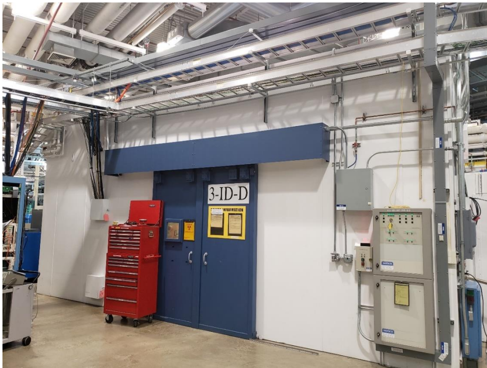
The hutch, door closed and during operation.
