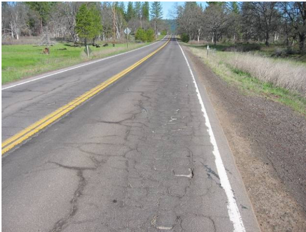
Consistent cracking on selected section
