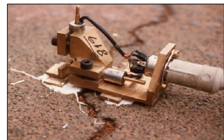
Crack activity measurement
