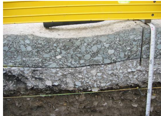
Close up view of distress (rut in underlying AC)
