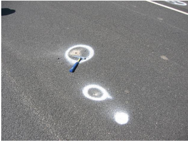
Poor quality construction - thickness control
