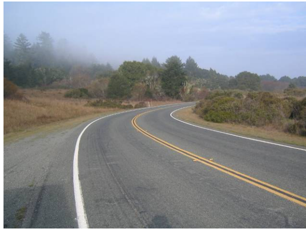
Consistent bleeding/stone loss on selected section
