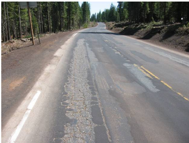
Inconsistent rutting and cracking
