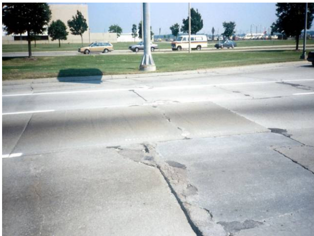
Inconsistent spalling, cracking, and faulting
