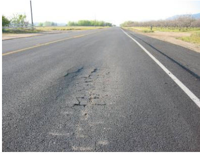
Surface distress in new overlay
