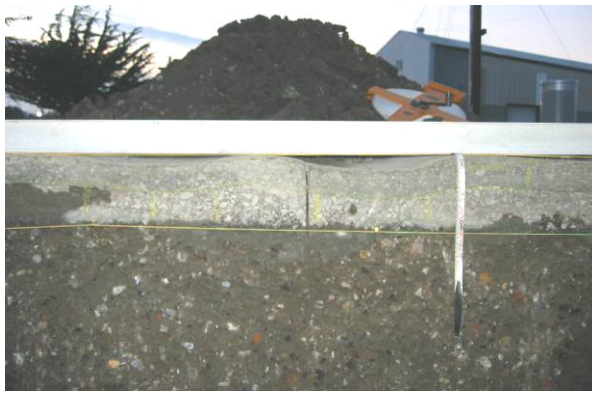
Note rutting in underlying AC layer.
