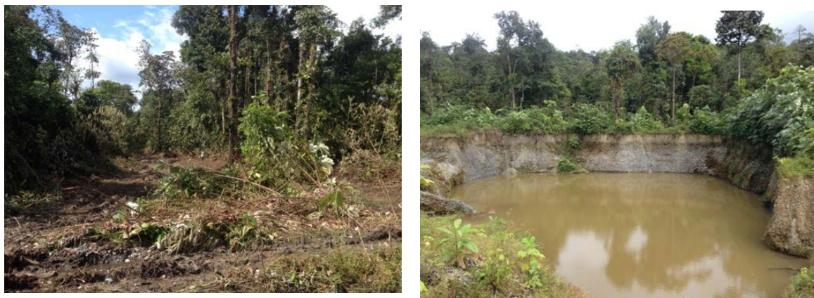
Figure 5.7. Mining in Los Cocos with excavators starts with clearing the land of vegetation (left), and then digging pits from which to pull and wash sediments. These are the pits that community members pan in while they are being dug out by the excavator, and water is being removed from them by a motor pump.
