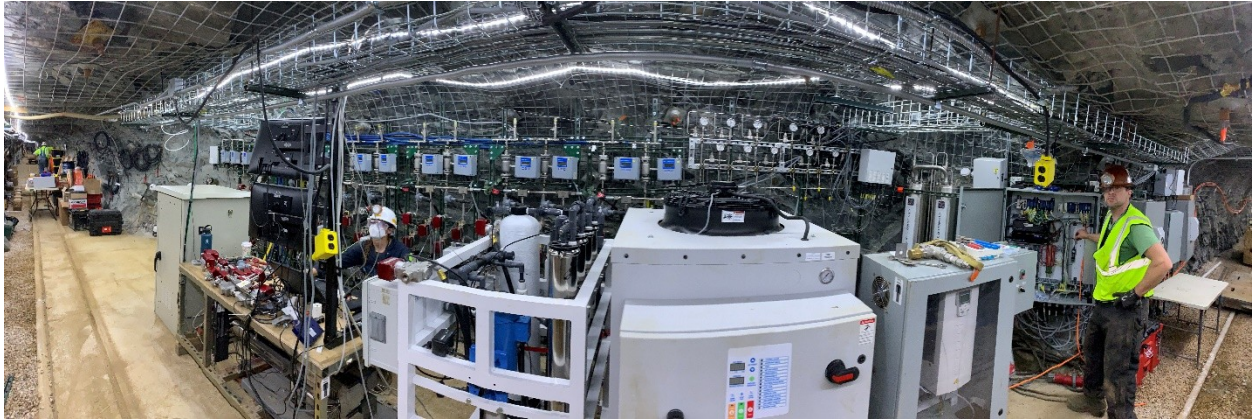
Figure 16: Panoramic of the system as installed on the 4100 level. Note the modular plumbing hung on the wall behind the other equipment and the control computer.
