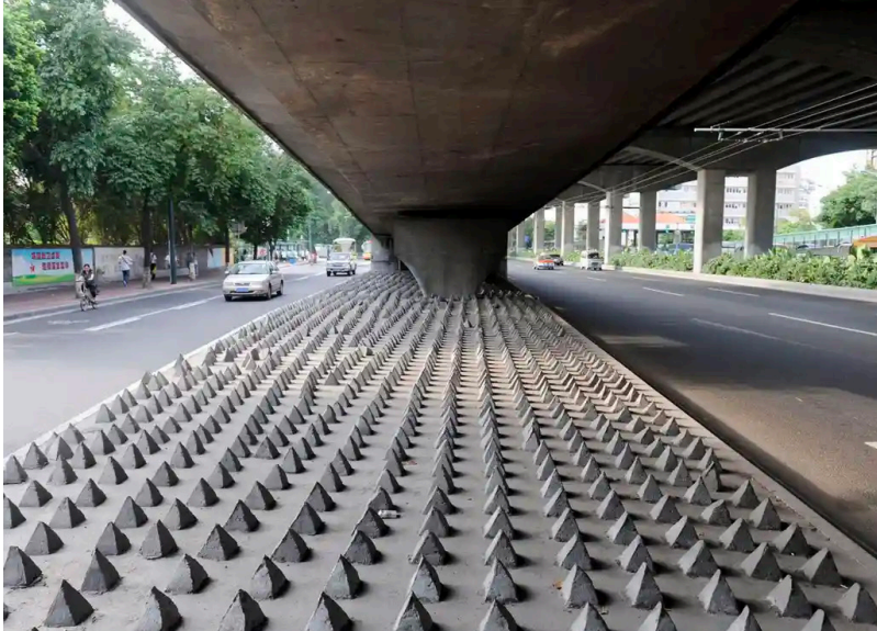
Concrete spikes under a road bridge in Guangzhou city, Guangdong, China (Reed, 2015)
