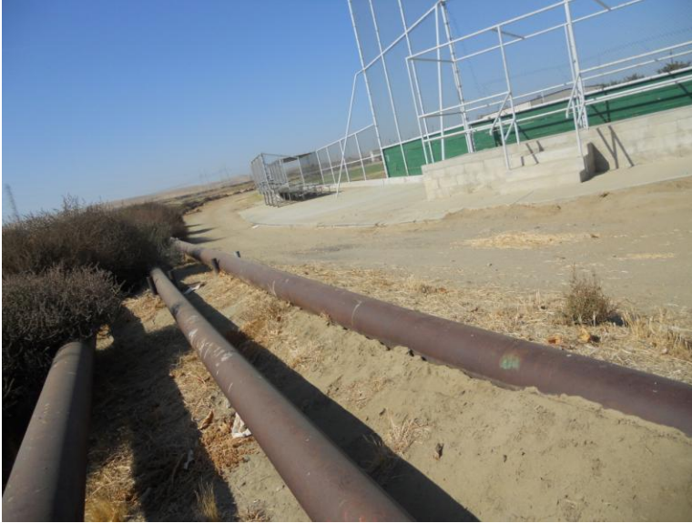
These pipelines run behind the playing field of the school. Photograph by Yalda Asmatey
