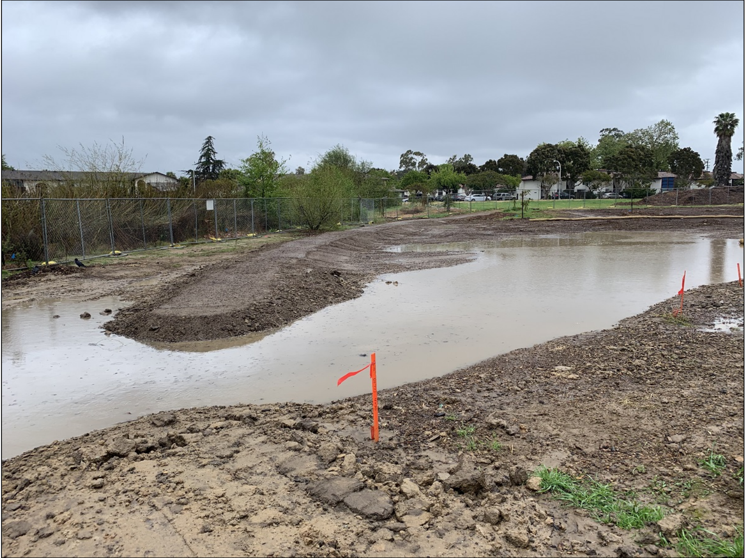
In this image, we see the foundation of the discovery trail and future location of a bridge over the bioswale, which is filled with run-off from recent rains.
