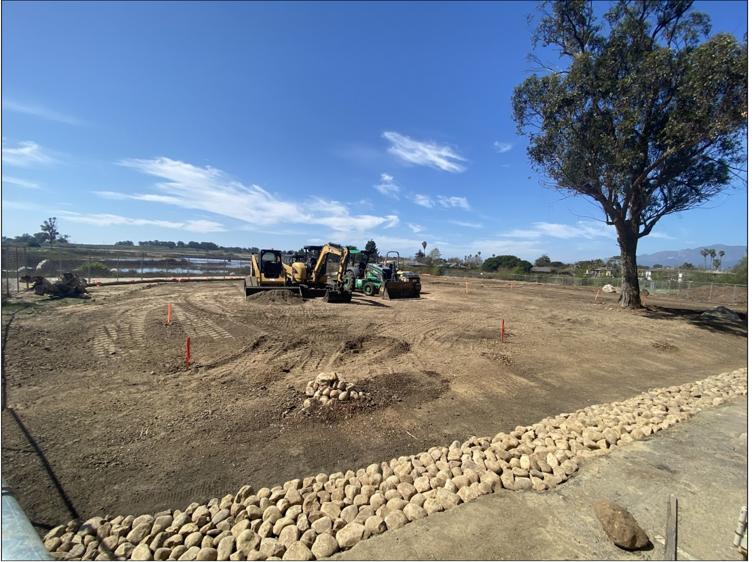
In this view of the Visitor Plaza construction site, we can see the rocks that form the foundation of a bioswale that will capture and filter run-off from the parking lot.
