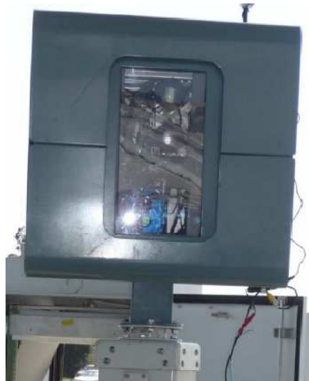
Figure 1 dtect Camera Installed at I-15
