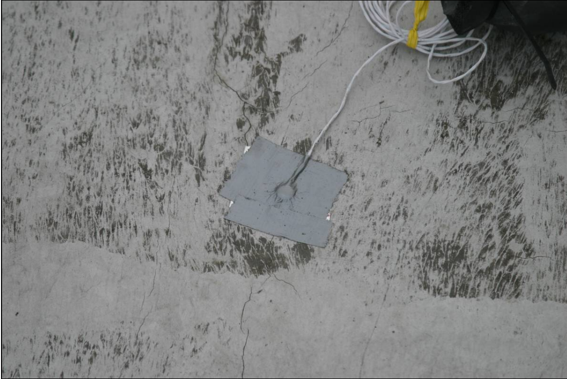
Figure 8. A close-up view of the roof surface temperature sensor location near the RTU before and after the white roof coating was applied. During late afternoon and early evening hours, the sensor was shaded by the south air temperature sensor towers and by the RTU.
