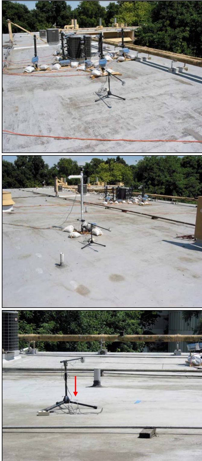
Figure 3. Views of the three roof reflectance measurement locations (before the white roof coating was applied): west of the test RTU, adjacent to the weather tower near the center of the roof, and near the north surface temperature sensor (marked by an arrow).
