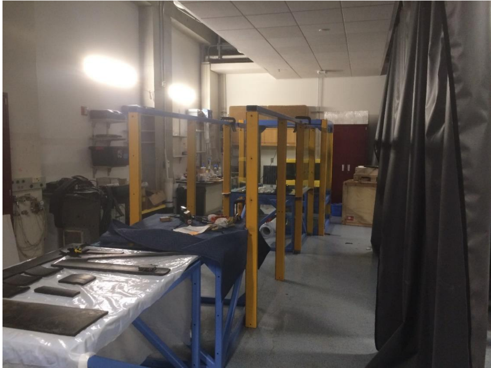
Figure 5.7a: Setup of the vertical members. This was done to guide the chassis modules and to aid in holding the vertical glass panels together once installed
