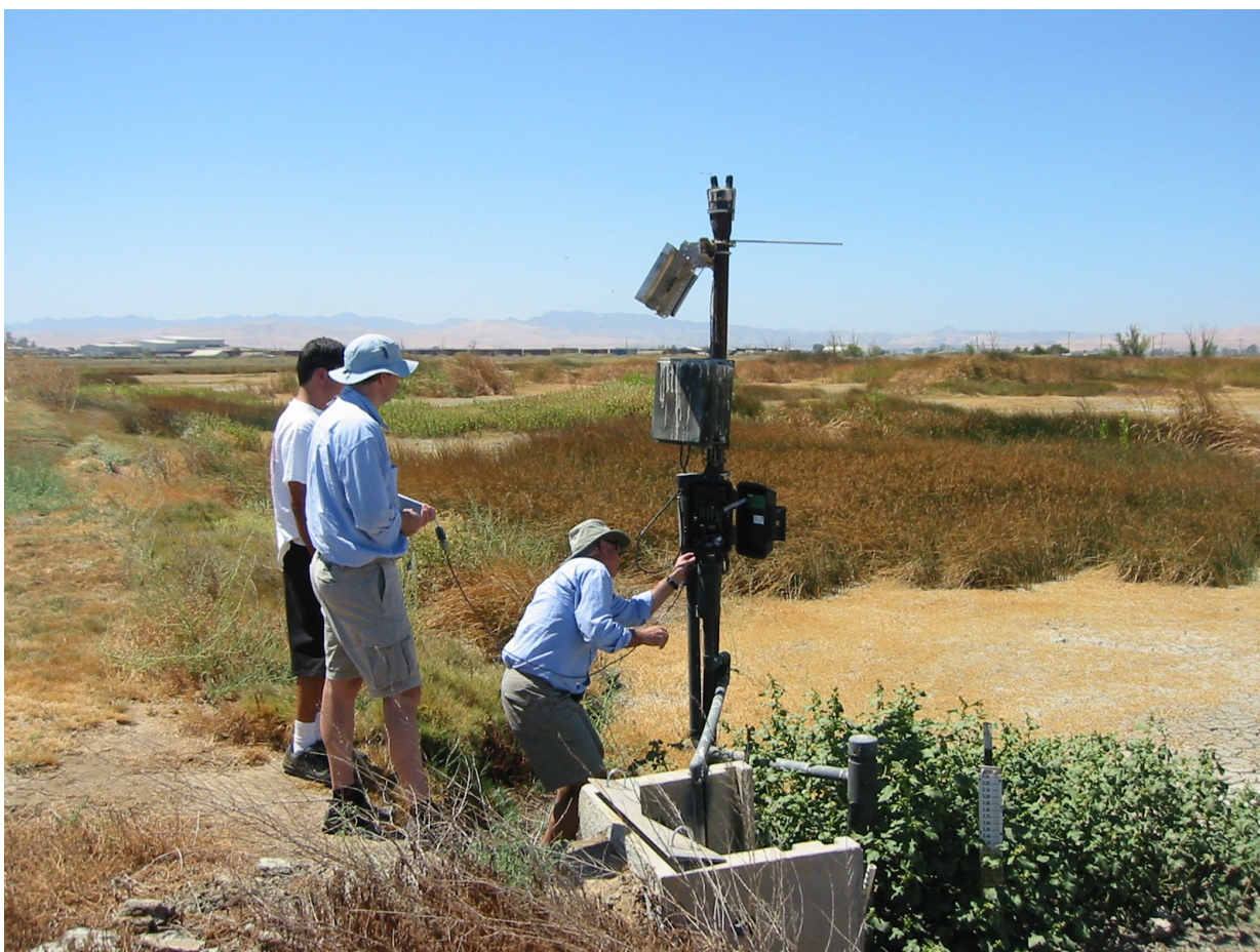
Figure 3.2. MACE USA President Mathew Campbell in the field with Tim Quinlan (sales rep), Ric Ortega (DFG) and Nigel Quinn (photographer) replacing the circuit boards in the Series III instrument boxes to restore output parameters (stage and velocity) and solve the decimal point placement issue .
